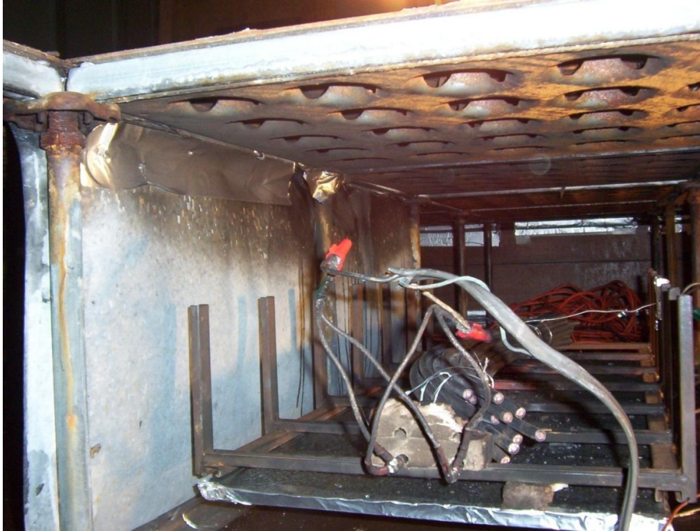
Figure 6. Cable bundle in sub-floor
