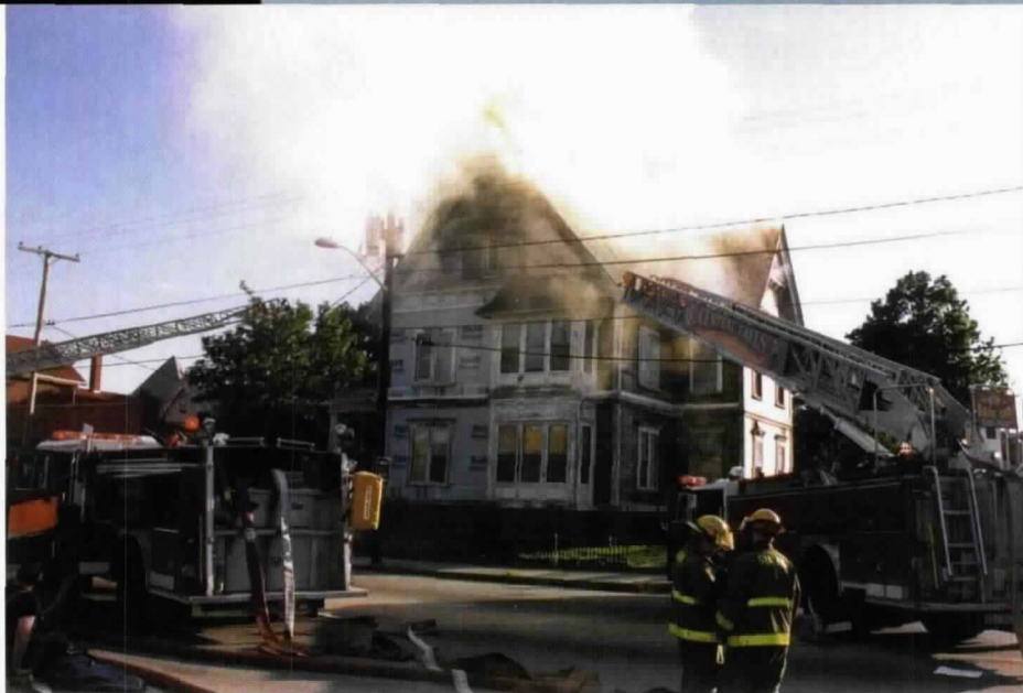
Youths began a fire in this vacant three-story Victorian mansion. The fire was set on the third floor and heavily damaged the building.
