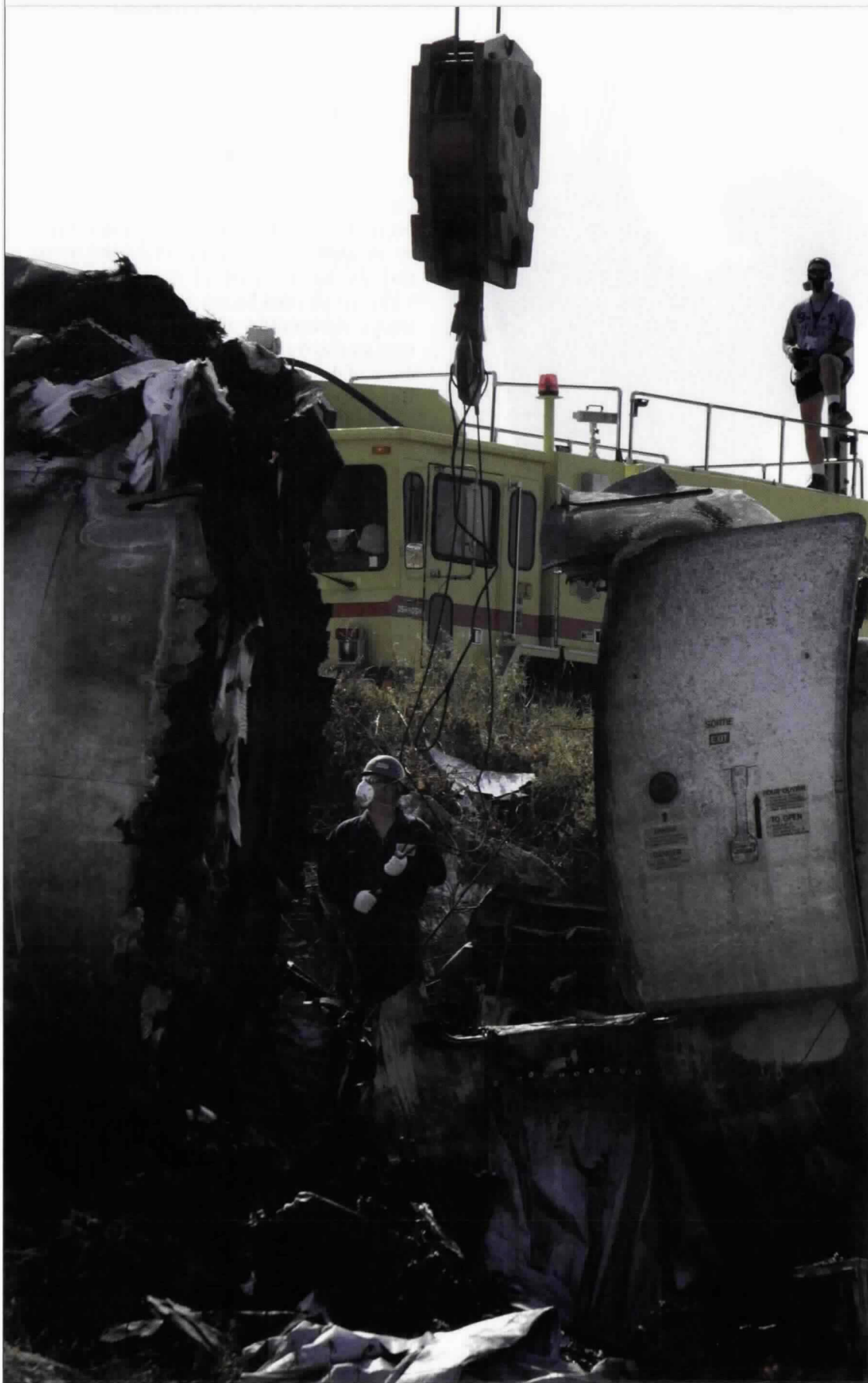
A firefighter watches over as a demolition worker attaches a crane to part of the fuselage of Air France flight 358 at Pearson Airport in Toronto.
