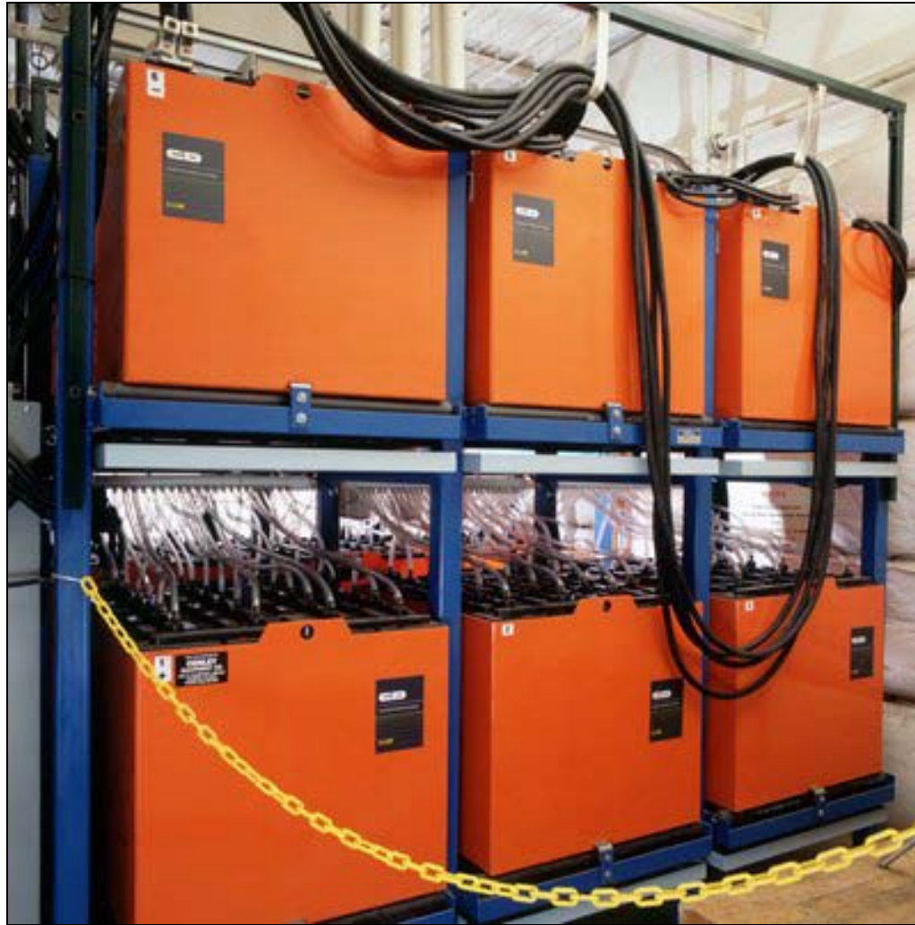
Battery Installation (for a Photovoltaic Solar Power System) (Issues: Distributed Energy Resources, Power Isolation/Shutdown, Jurisdictional Scope, etc...)
