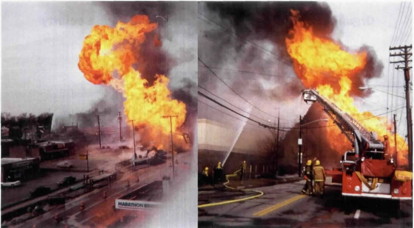
A construction crew installing a storm drain at an intersection was trying to find a bypass valve when the valve's flange cover ruptured, which led to a natural gas fire. There were no injuries, but the explosion damaged 10 structures and 21 vehicles.
