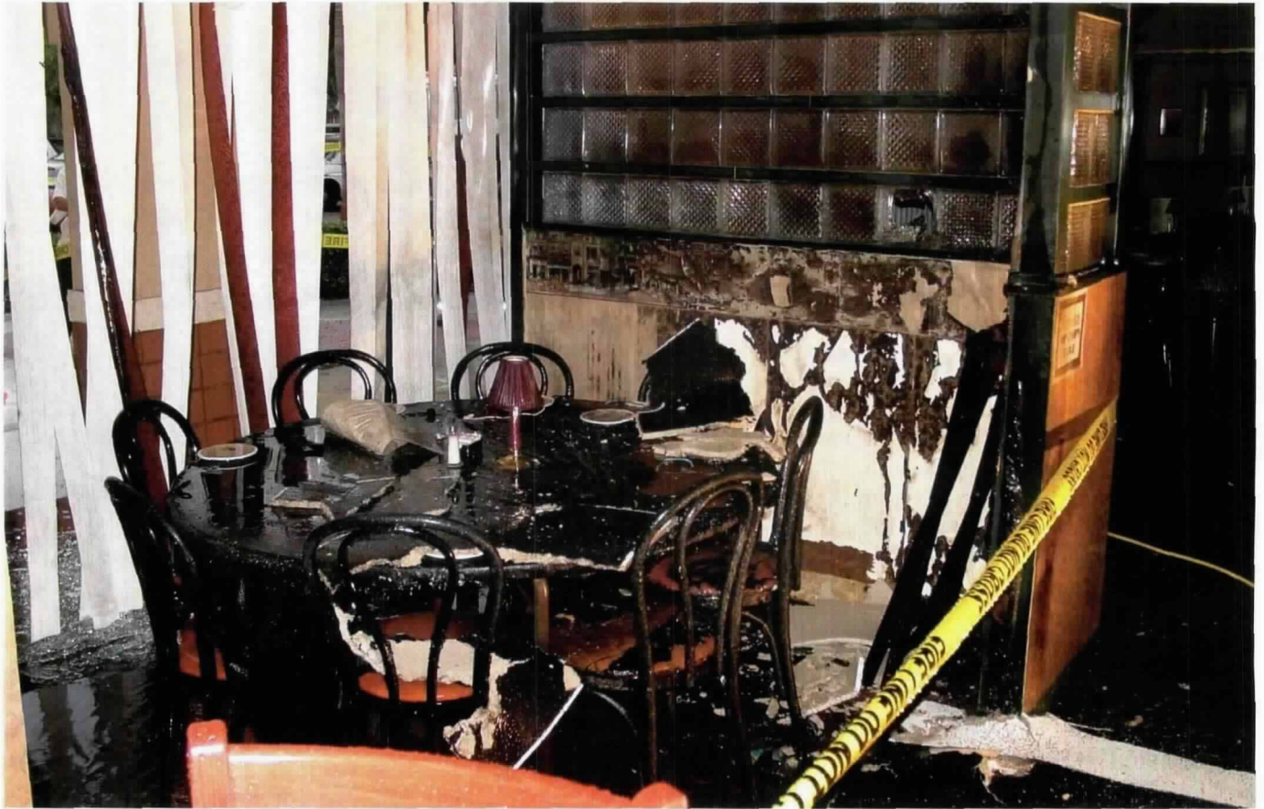
Three Molotov cocktails were thrown into a restaurant through the front window, but a single fire sprinkler quickly extinguished the fire.
