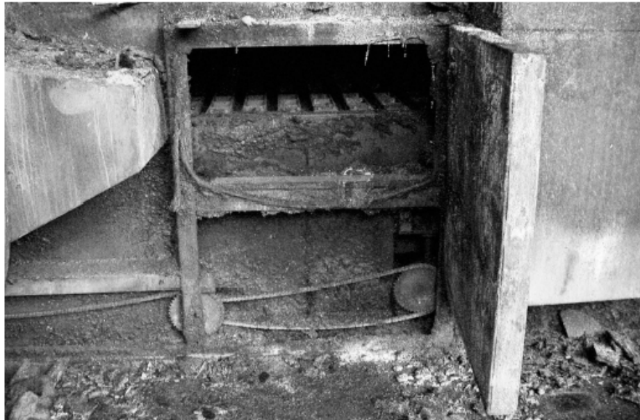
Figure 13. Interior of line 405 oven.
