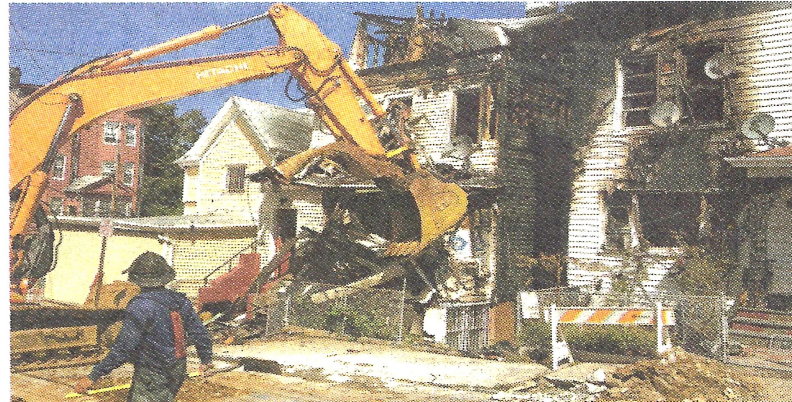
Workers demolish 103 Webster Ave. in Yonkers. Sunday's four-alarm fire damaged the building.
