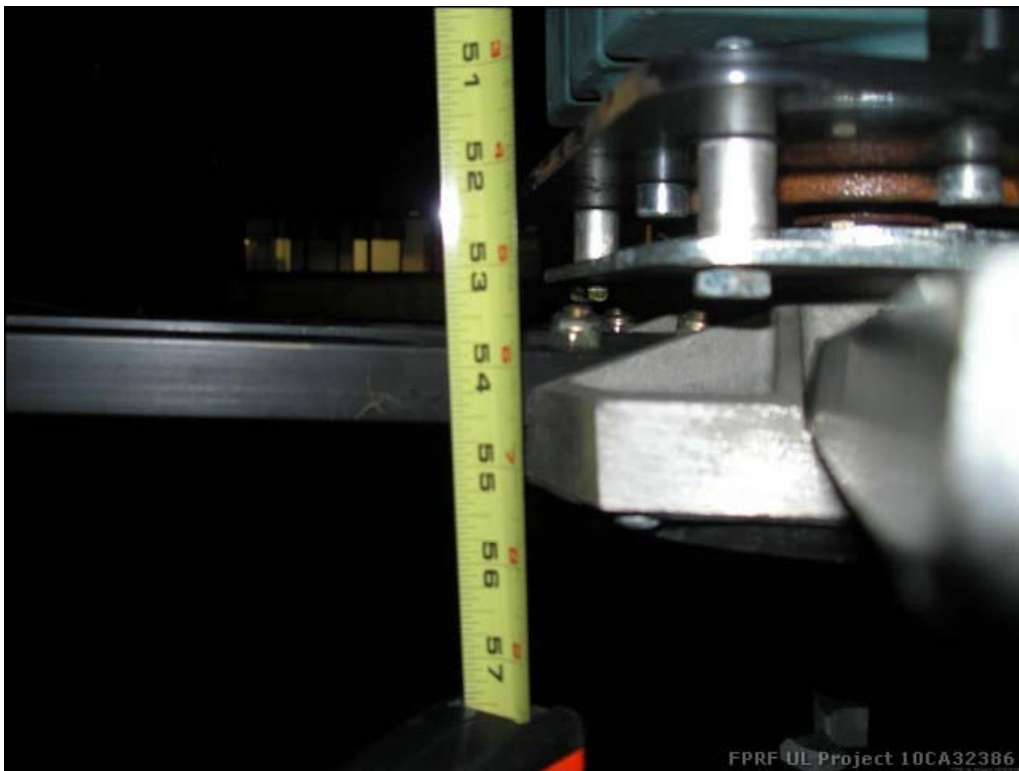
Figure 34 HVLS Fan Installation
