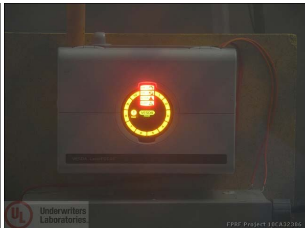
VESDA Control Panel (in full alarm after 01:28)
