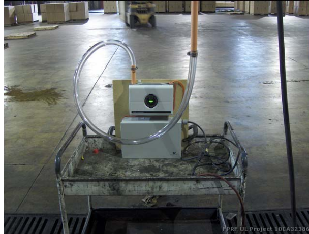
Figure 9 VESDA Control Unit
