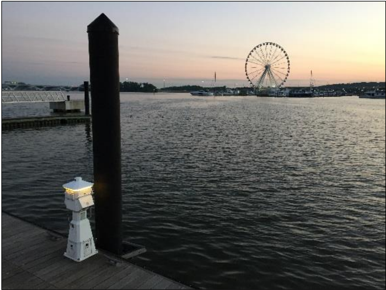
Figure 7: Typical Electrical Installation at a Marina
