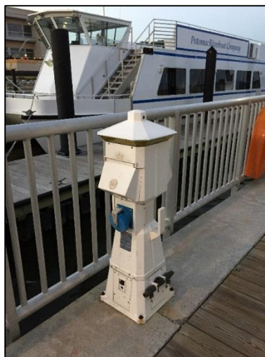
Figure 1: Typical Electrical Installation at a Marina
