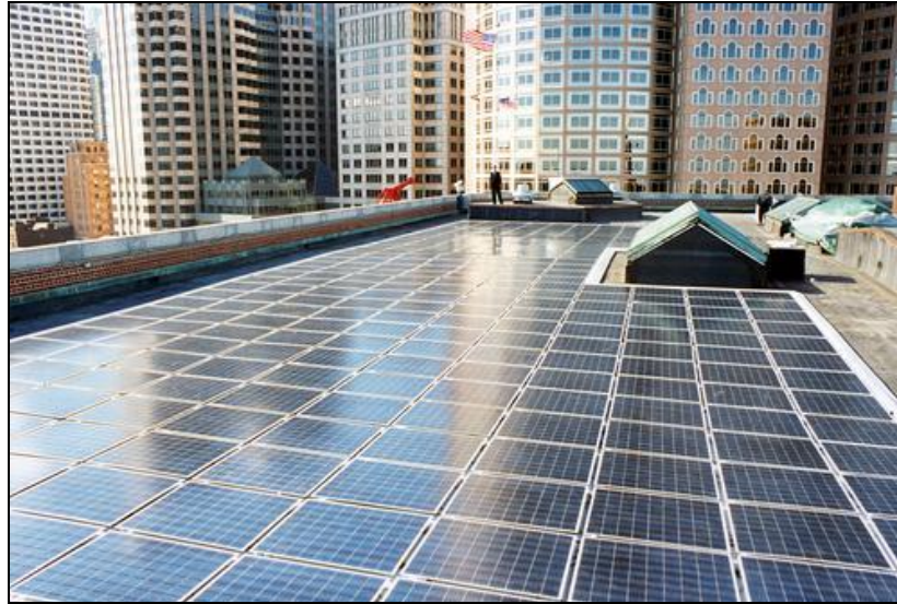
Figure 2-5: Example of a Large Solar Power Commercial Installation (Photo courtesy of NREL Photographic Information Exchange)
