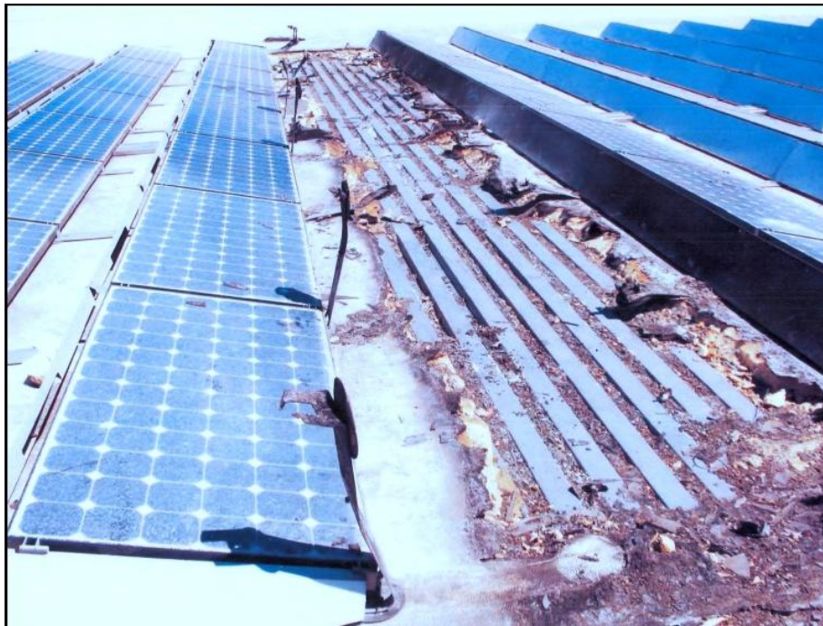
Figure 2-12: Fire-Damaged Array in April 2009 CA Incident 46
