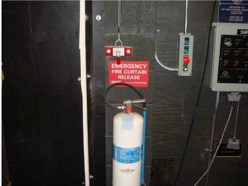
Figure C12 – Manual means of fire safety curtain release provided adjacent to proscenium opening
