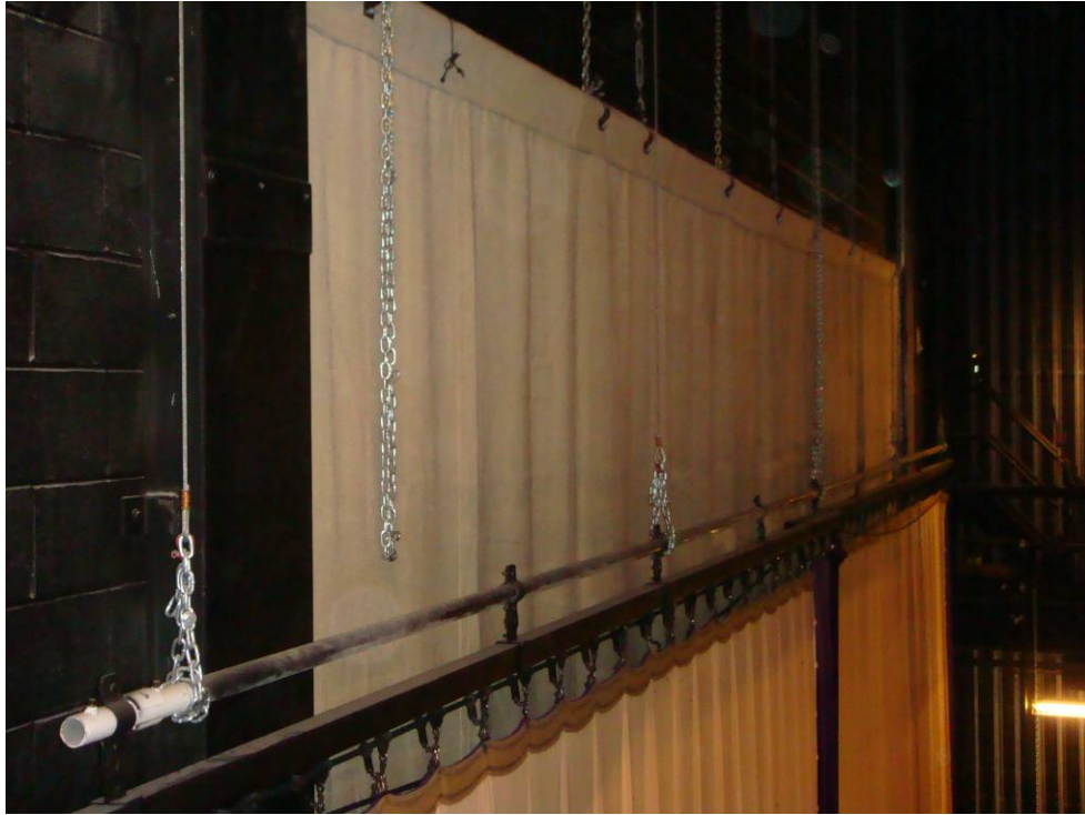
Figure C11- Fire safety curtain at gallery level
