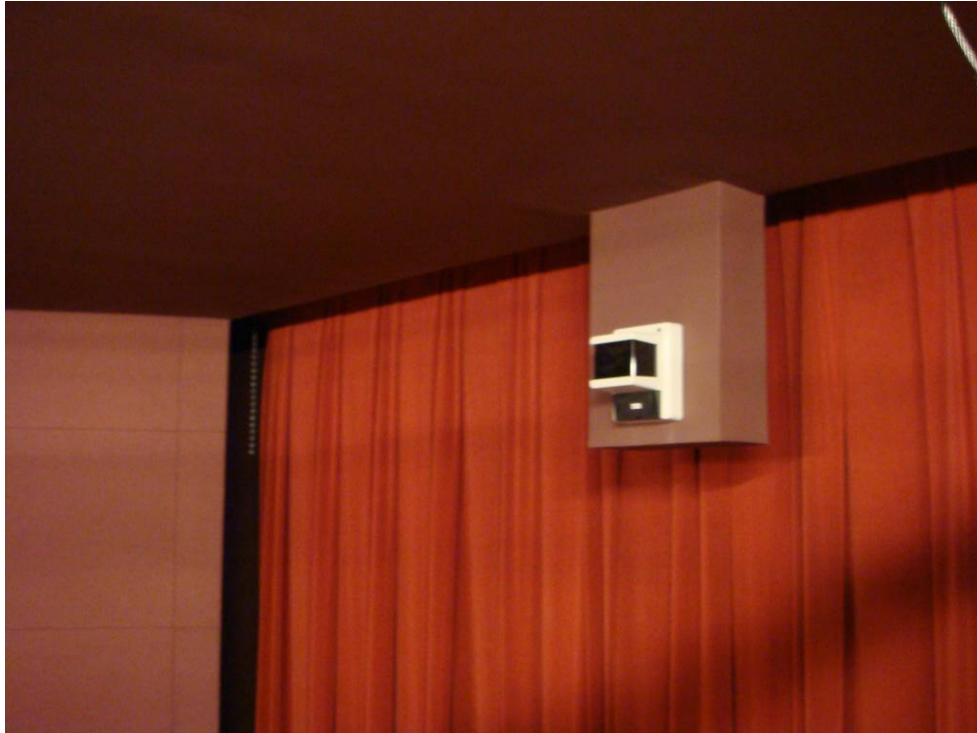
Figure C3 - Projected beam smoke detector provided in seating area
