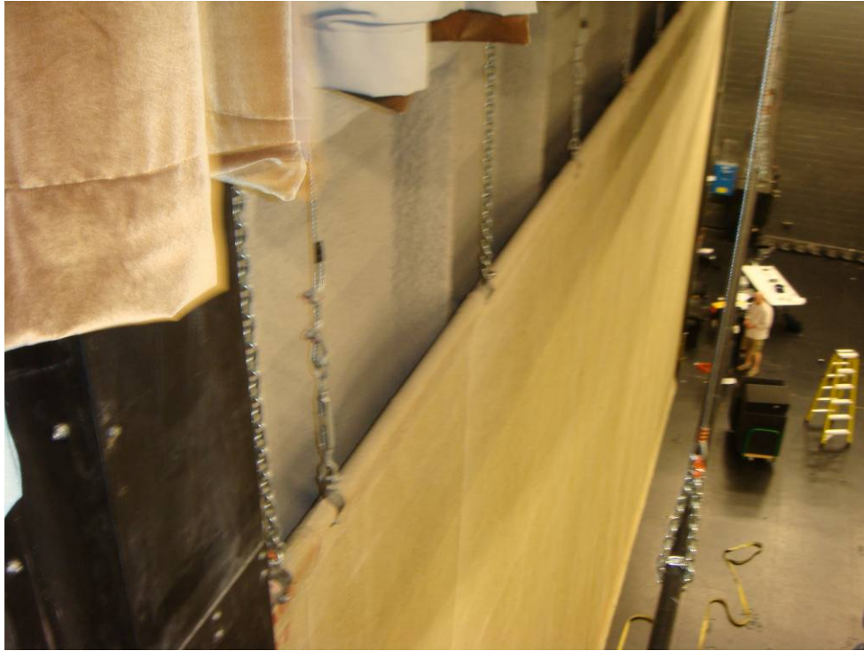
Figure C21– Top of Fire safety curtain at gallery level
