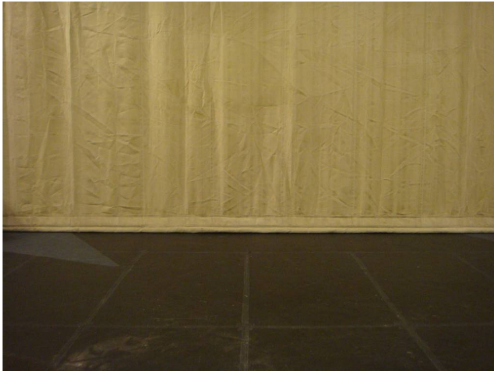
Figure C10- Bottom of fire safety curtain after deployment
