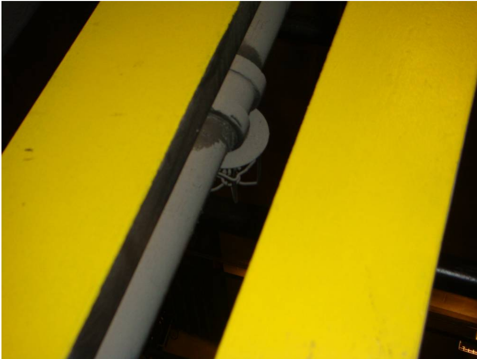
Figure C18– Sprinkler under gridiron
