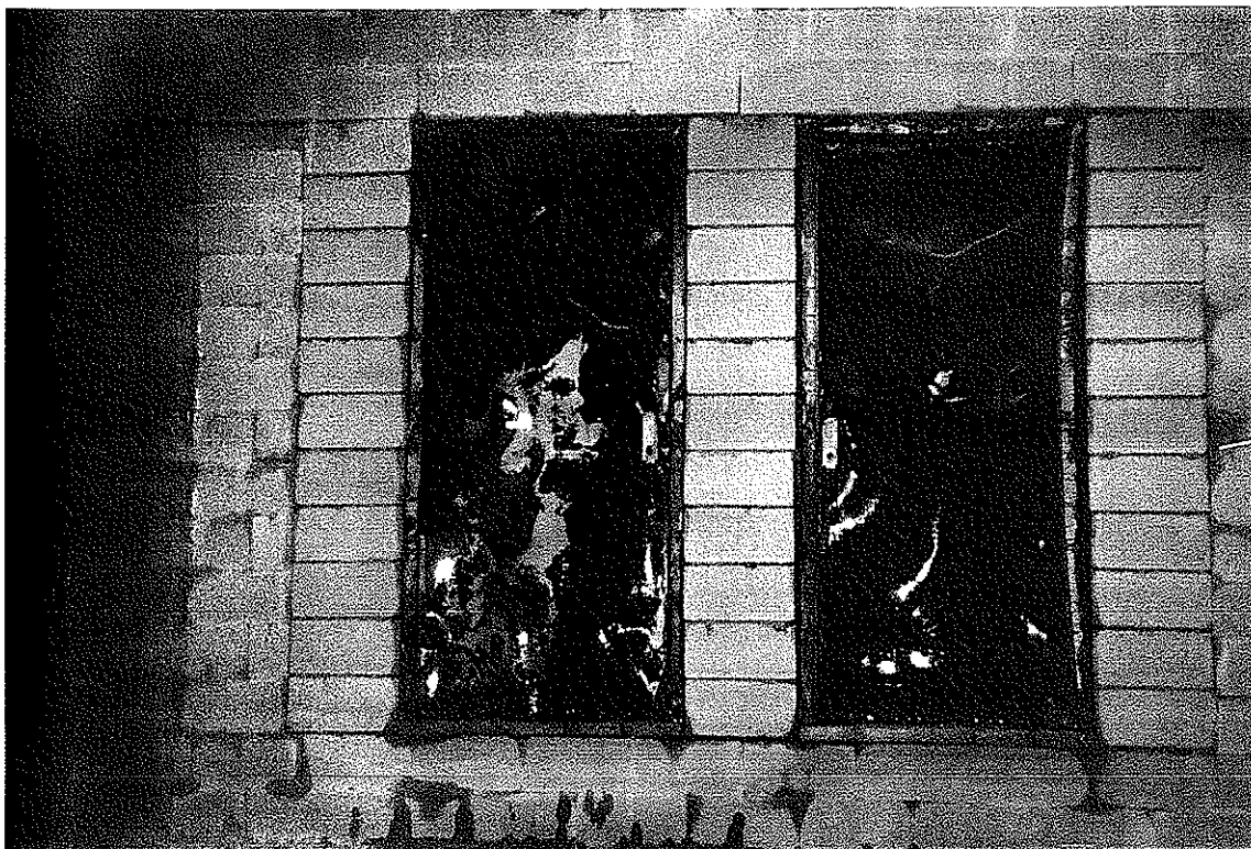
EXPOSED SIDE AFTER HOSE STREAM TEST
