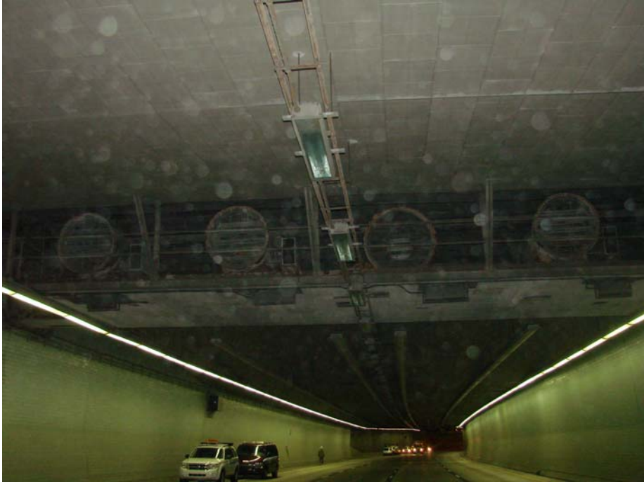
Figure 2.3. Jet fan system in Tube A of the Carré-Viger Tunnel
