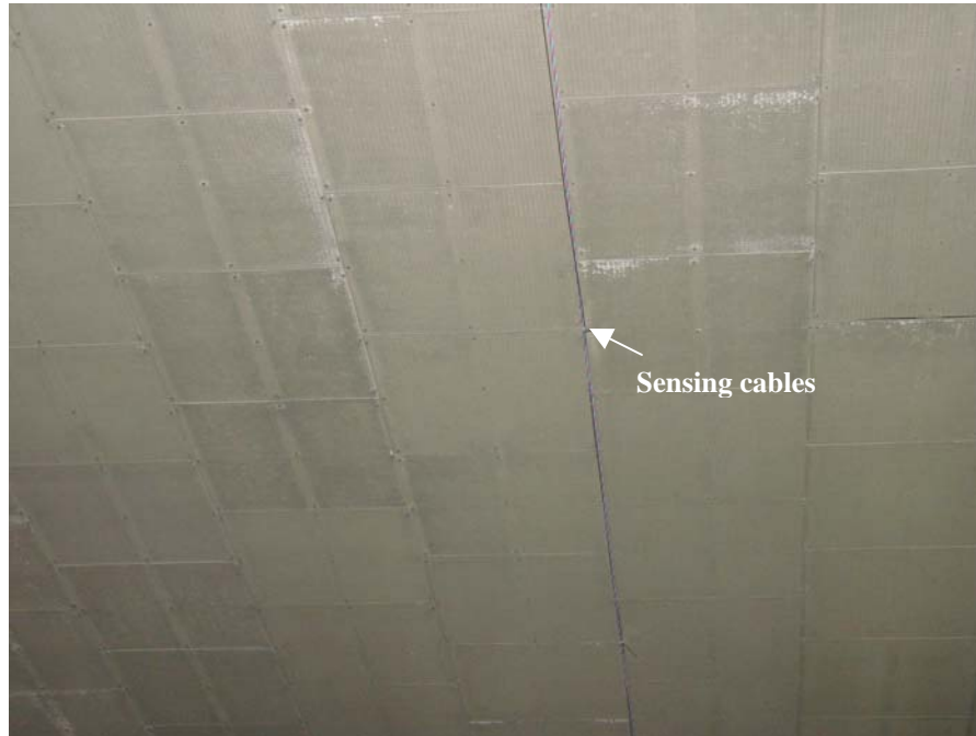
Figure 3.2. Photograph of linear heat detection systems
