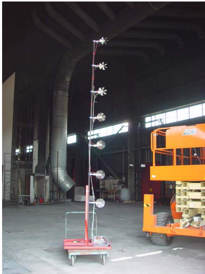
Figure 6.2. Photograph of the air velocity meter tree
