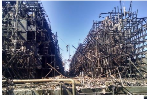
Figure 23 Damaged cooling tower.
