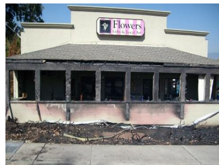
Figure 25 Damaged commercial business.
