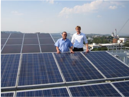
Solar photovoltaic installation on the roof of El Salvador's primary electricity generator
