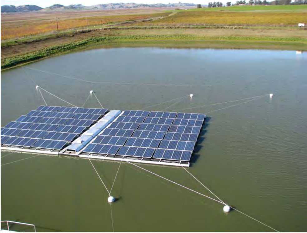
38kW Demonstration Installation of 2010 Floatovoltaics®
