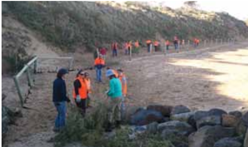
Queenscliff Narrows and Gordon TAFE stabilising works Photo: Matt Crawley, Bellarine Catchment network.
