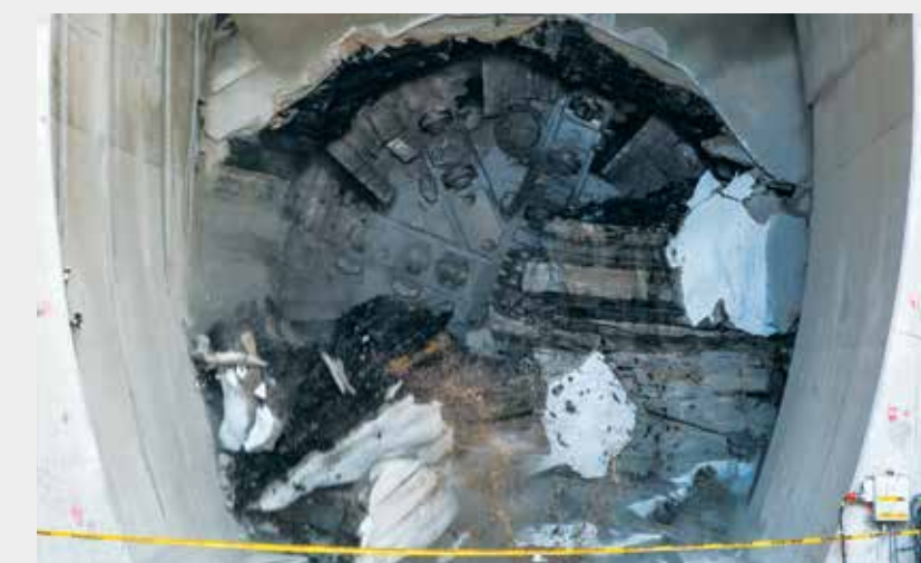
Size and scale of a TBM in action at Norwest in March 2015
