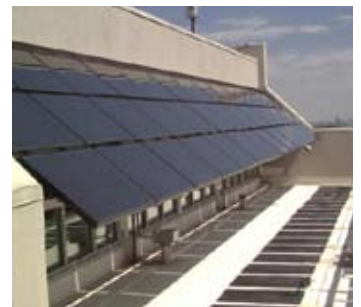
Inclined PVs with windows
