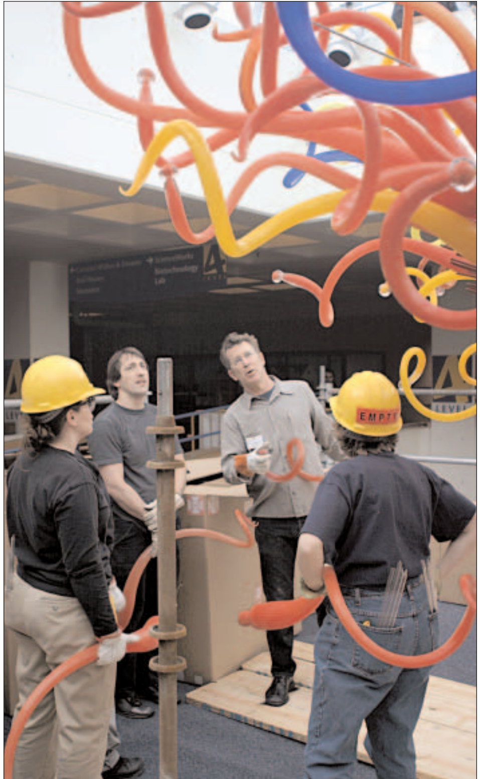
The Chihuly team and museum staff members work together to construct the Fireworks of Glass Tower .
