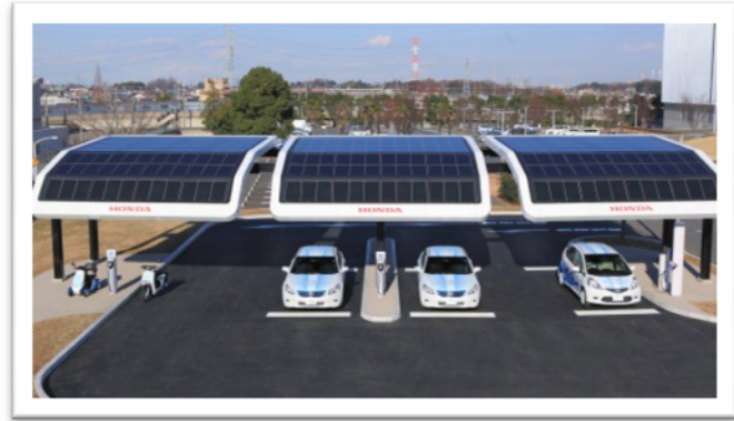
Figure 7-6: Honda Solar Powered EV Charging Station Source: http://www.gizmag.com/honda-solar-powered-ev-charging-station/17326/
