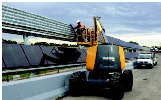
Figure 7-2: PV Panels on Solar Wall on Melbourne's M-80 (Western Ring Road)
