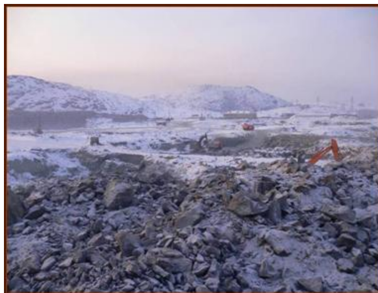
Figure 3. Preparation of grounds – explosions, rock and soil removal. Construction site in February 2005
