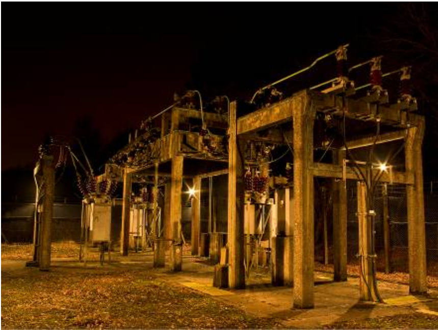
33kV outdoor HV raft
