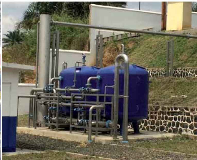
Drinking water treatment plant, 50 m 3 /h (Tonga, Cameroon)
