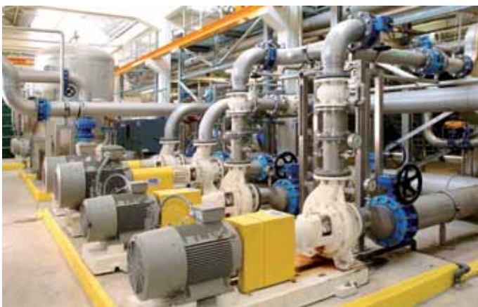
Drinking water treatment plant and pumping station, 800 m 3 /h (Jambes, Belgium)
