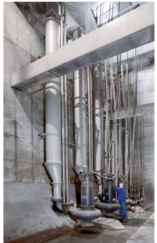
Pumping station of wastewater (Ampsin, Belgium)
