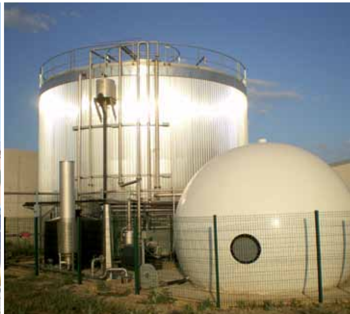
Methanization (Casseneuil, France)
