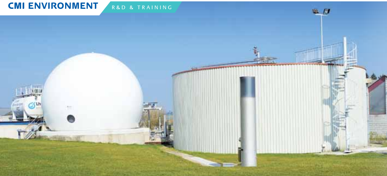
Sludge methanization (Marche, Belgium)
