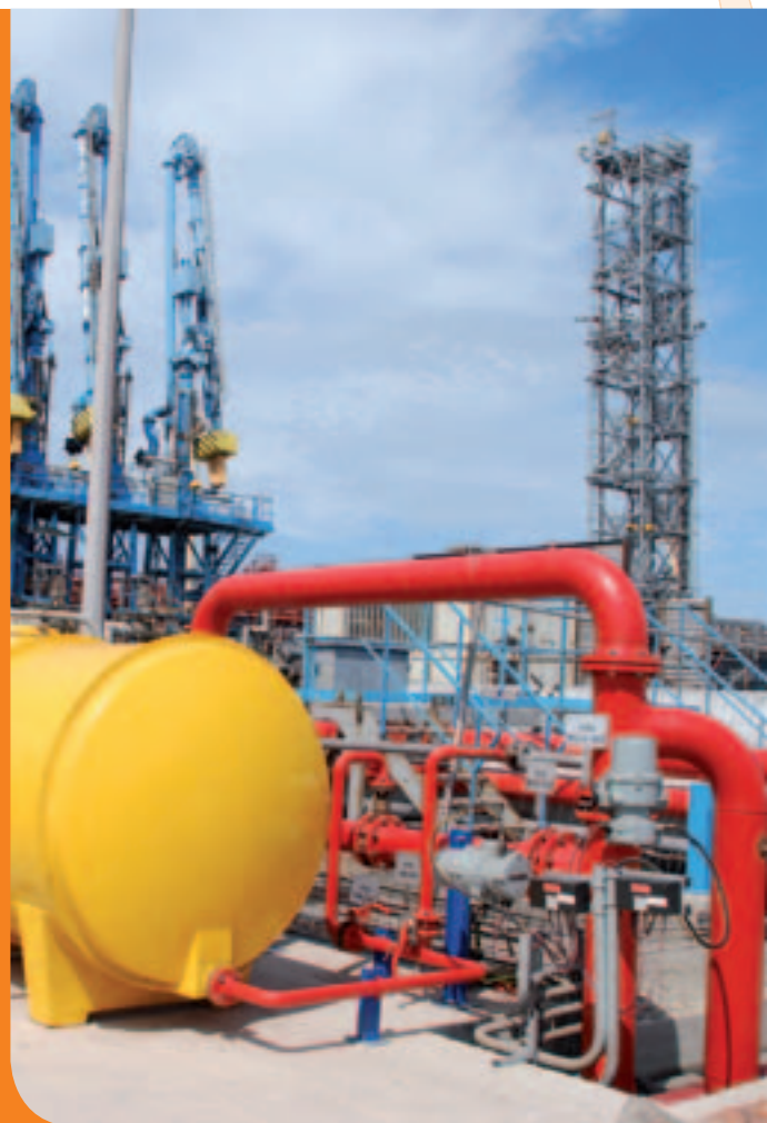
► In 2011 CMI Services installed several kilometers of pipework and framework in the Fos-sur-Mer (France) oil terminal. Here a view of its fire network.
