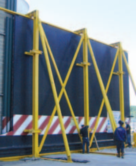
► In 2011 CMI Services developed its on-site machining capacities. Here, repairs to a machine room door on the EDF nuclear plant at Cattenom (France).
