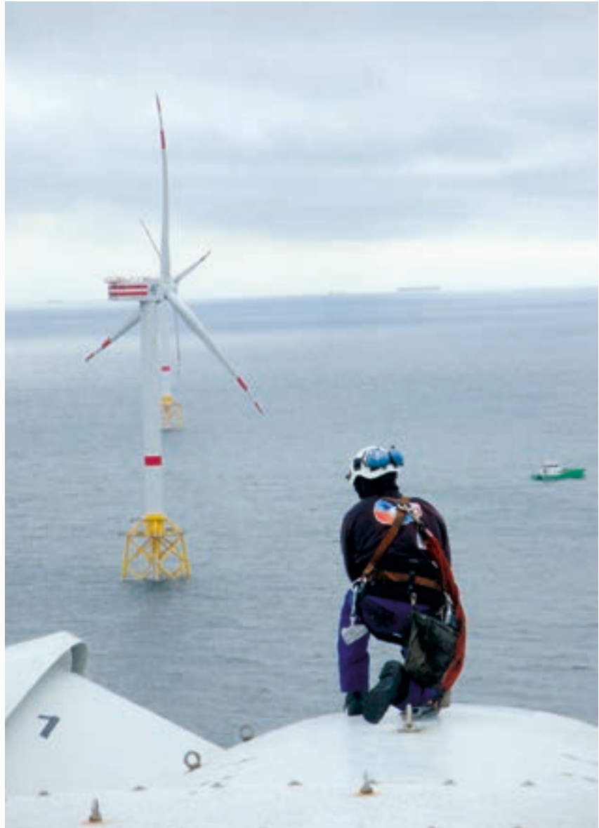
▲ Whether through its work on hydropower facilities, on boilers or, as shown here, on wind turbines, energy maintenance activities remain a sound value within the offering of CMI Services.
