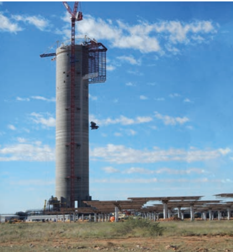
▲ Installed at the top of a 200 m high tower, the first CMI thermo-solar boiler will equip a 50 MWe power plant. The next CMI boilers of this type will be suitable for power stations which are five times more powerful.
