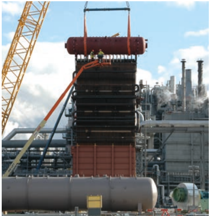
▲ The technical quality of CMI Energy's industrial boilers makes them particularly suited for use in the petrochemical sector.
