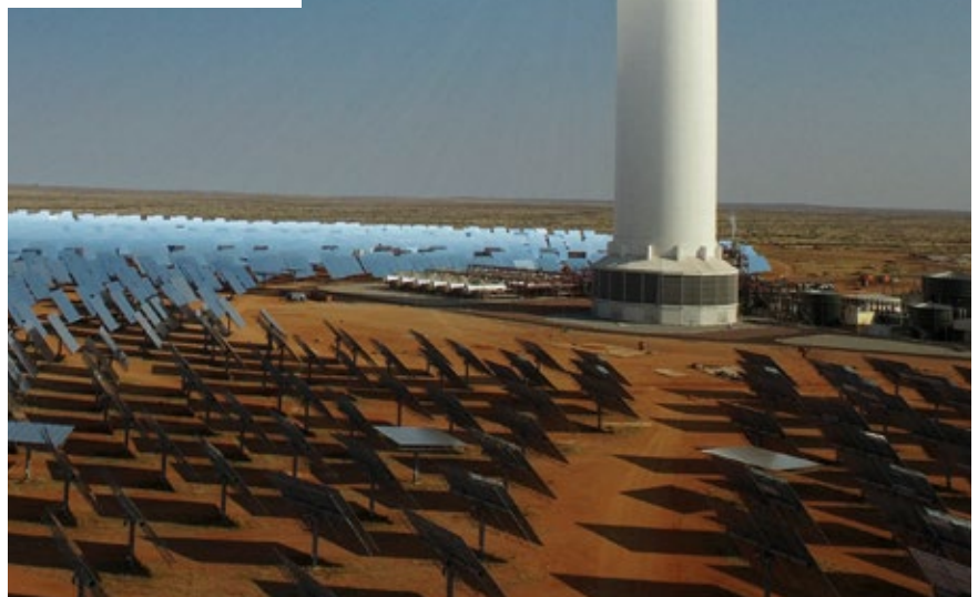
CMI designed and supplied the thermo-solar receiver for the Khi Solar One (South Africa) power plant, which entered service in 2016.
