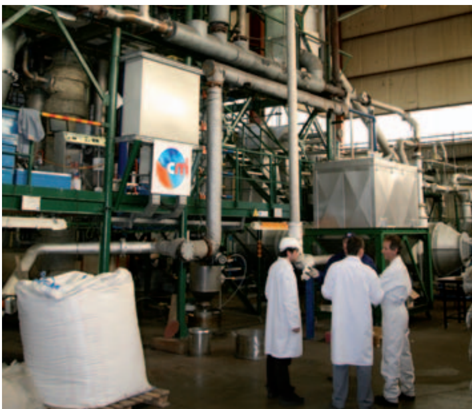
The pilot installation of the Nesa Solutions multiple hearth furnace is decisive in fine tuning the processes of its customers, irrespective of their field of application (biomass, magnesia, carbonated minerals, electronics...).
