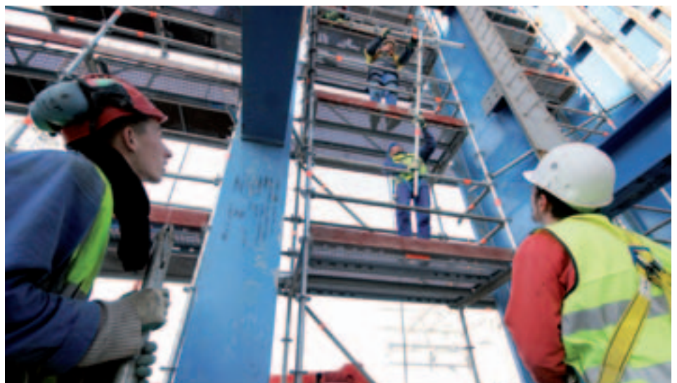
CMI Energy's proactive approach to safety on erection sites is hailed by all European energy customers.
