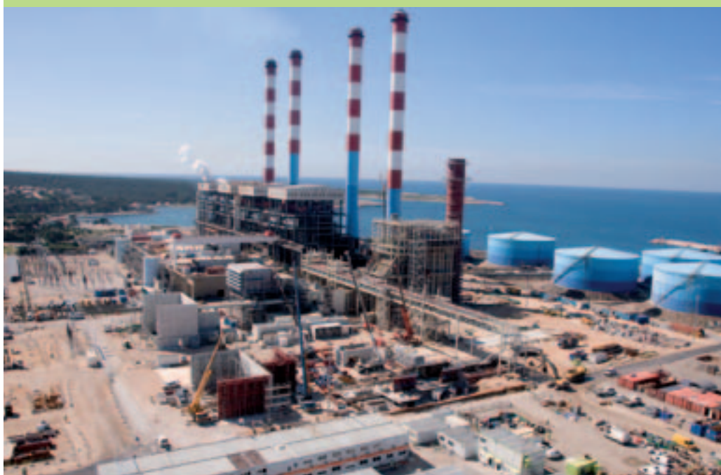
In 2010, CMI Energy erected thirty boilers throughout the world, 18 of which were commissioned.
