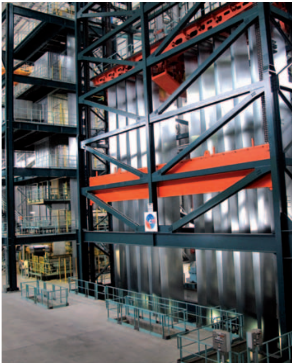
The new galvanising line of the Italian steelmaker Riva, one of the most sophisticated lines in the world, integrates the range of mechanical, thermal and chemical technologies of CMI Industry.
