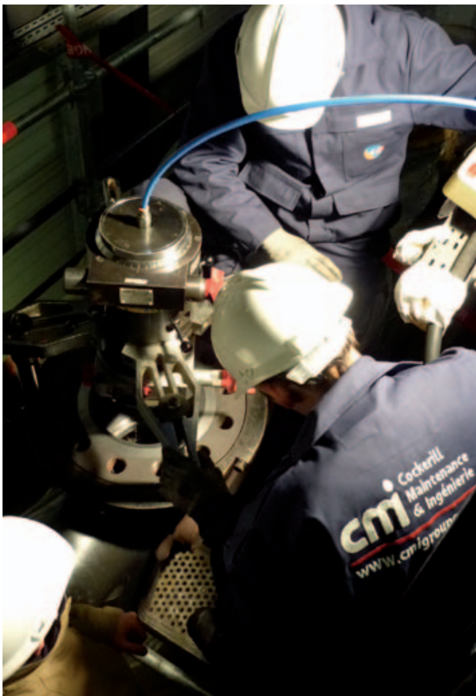
The work of CMI Services brings together local services and specialised technical interventions.
