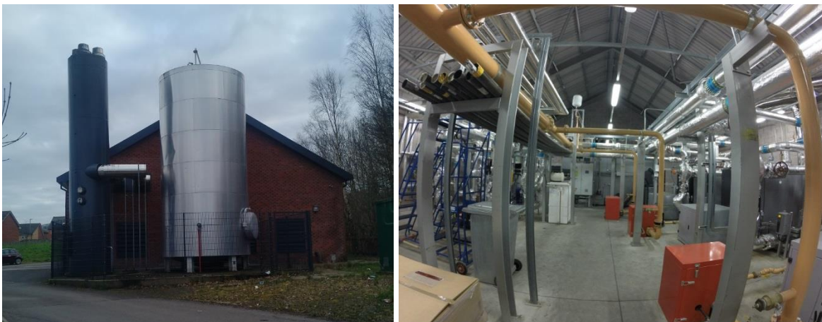
Figure 6.13: Picture of the thermal storage with 50,000 liters capacity (left) and the boiler house (right)
