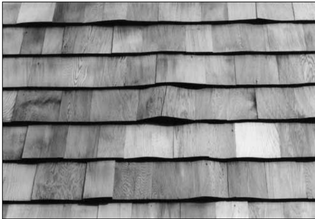
Figure 7. Buckling of shingles installed with insufficient gap.
