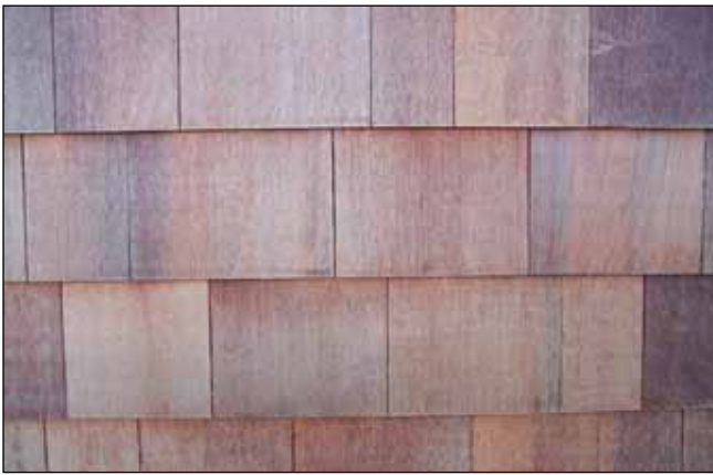
Figure 13. Shingles treated with tinted water-repellent preservative.
