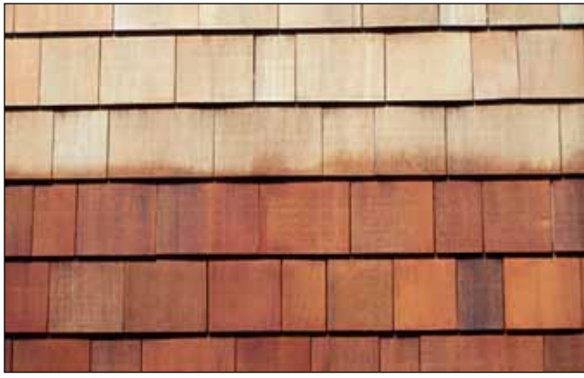
Figure 14. Semitransparent stain application to shingles that were let weather for about two years. NOTE: The stain application was not done correctly. The painter allowed stain to partially coat the bottom of the course of shingles directly above the stained portion. When the shingles above are stained, there will be a lap mark.
