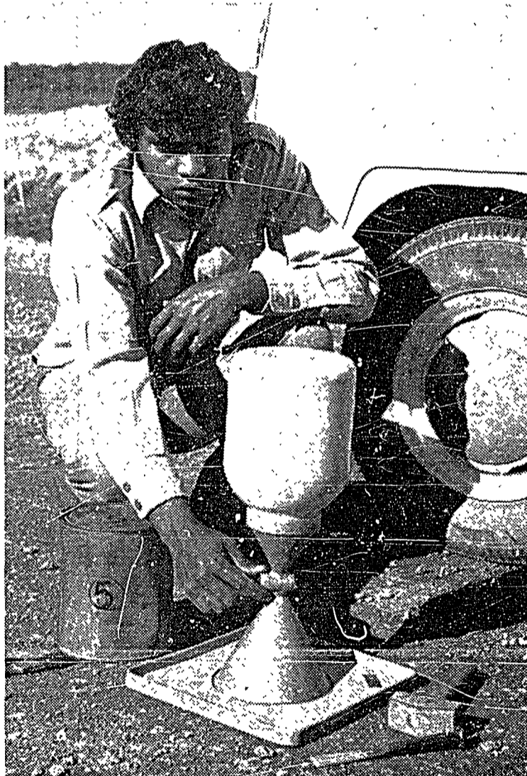
Right: Before sealing the four-mile-long site access road with asphaltic concrete, many samples were taken for compacted dry density tests of the road pavement.
