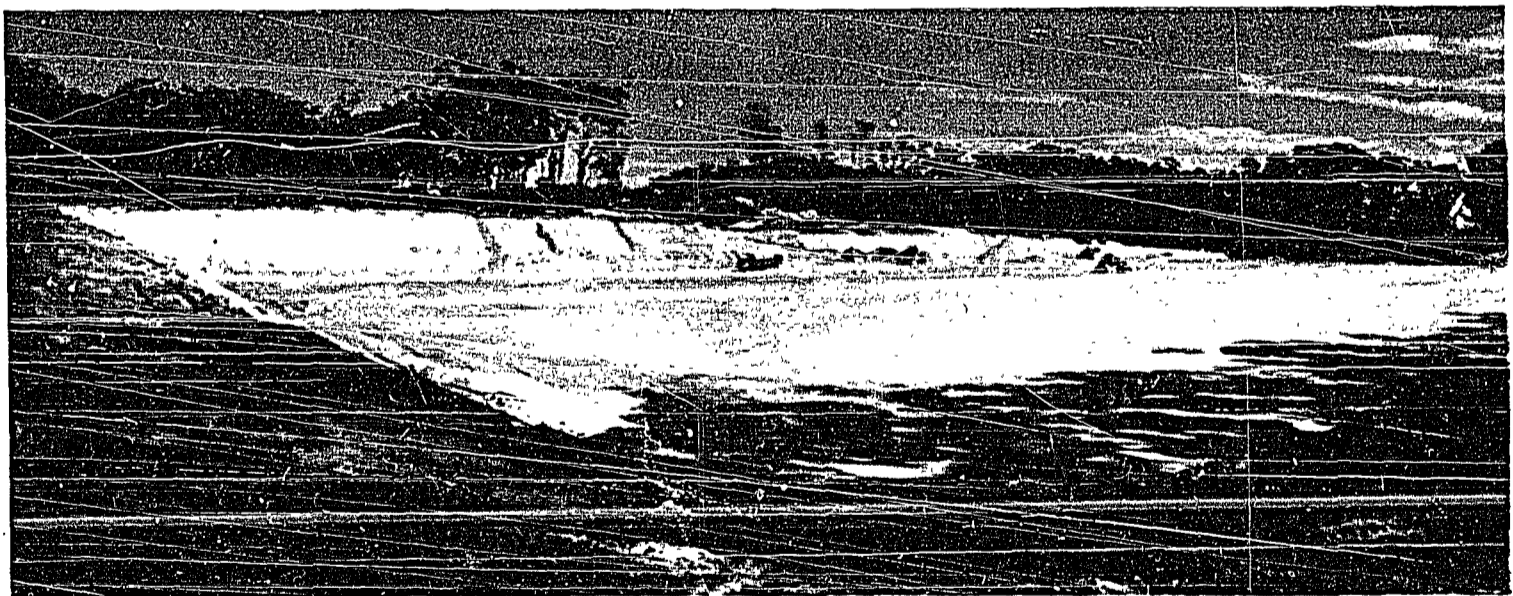
Initial excavation of the 850 ft x 550 ft site of the 500 MW nuclear power station. The area has been excavated to a working level of 14.5 ft above mean sea level. Top soil has been stockpiled for future landscaping on completion of the station. Excavation of the rock provided foundation material for the four-mile-long access road.
