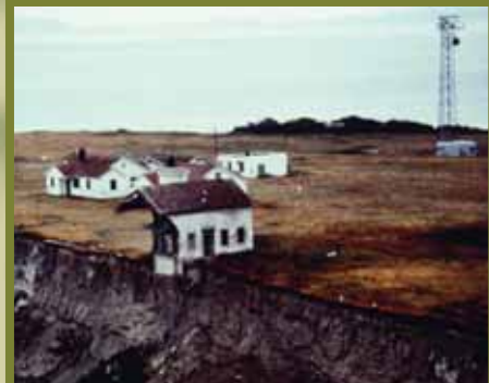
This image shows that a large portion of the lighthouse structure, which is the building to the right, has already fallen over the bluff. In the background you will see the skeleton tower, which became the new Smith Island Lighthouse.
