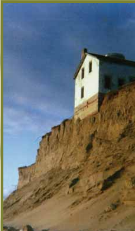
There is not much holding the lighthouse structure on the island in this 1975 photo taken by Coast Guard keeper Chris Donner. Notice that the entire foundation is exposed.
