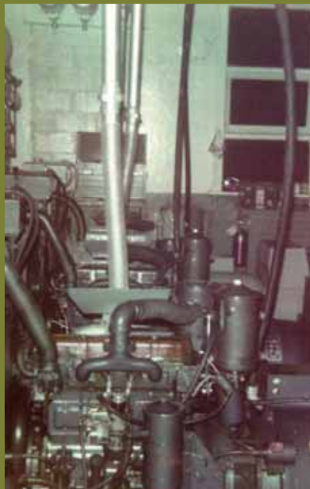
The generator room on Smith Island Light Station as it appeared in 1974. Photo by Chris Donner.
