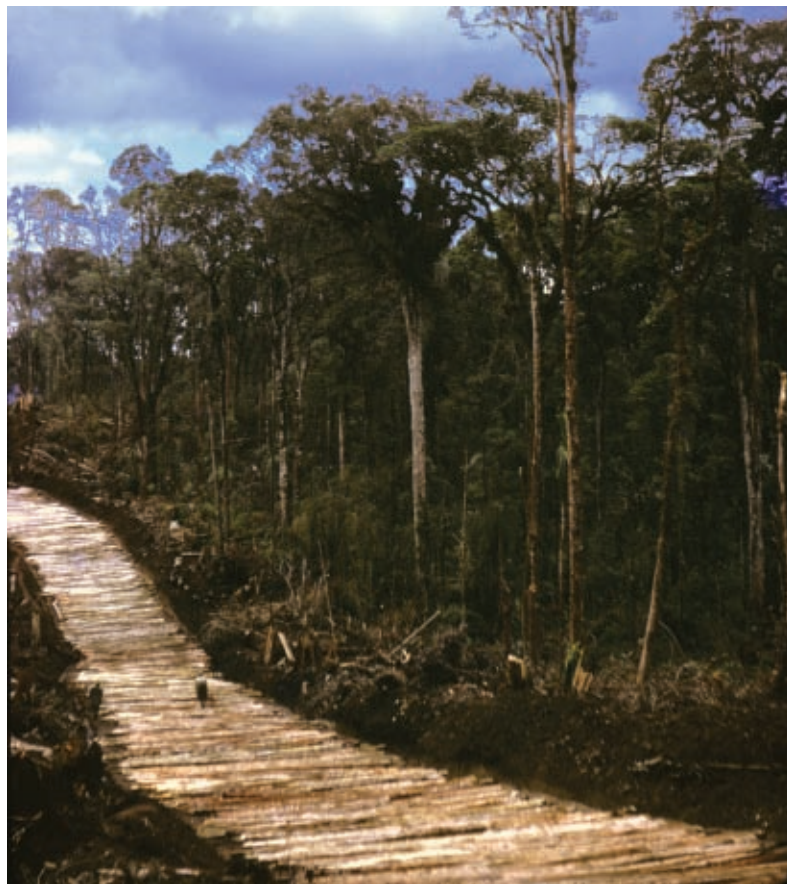
Plate 5: Logging in Nothofagus forests on Mt Giluwe. Note the extensive utilisation of felled trees in the 'cording' of the roads due to very muddy terrain. A person is visible in the middle of the road.
