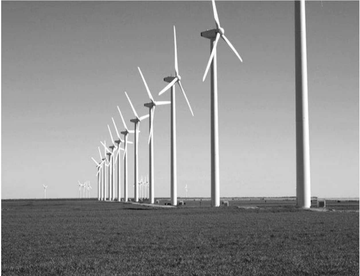
Brazos wind farm, Fluvanna TX, 160 1 MW wind turbines
