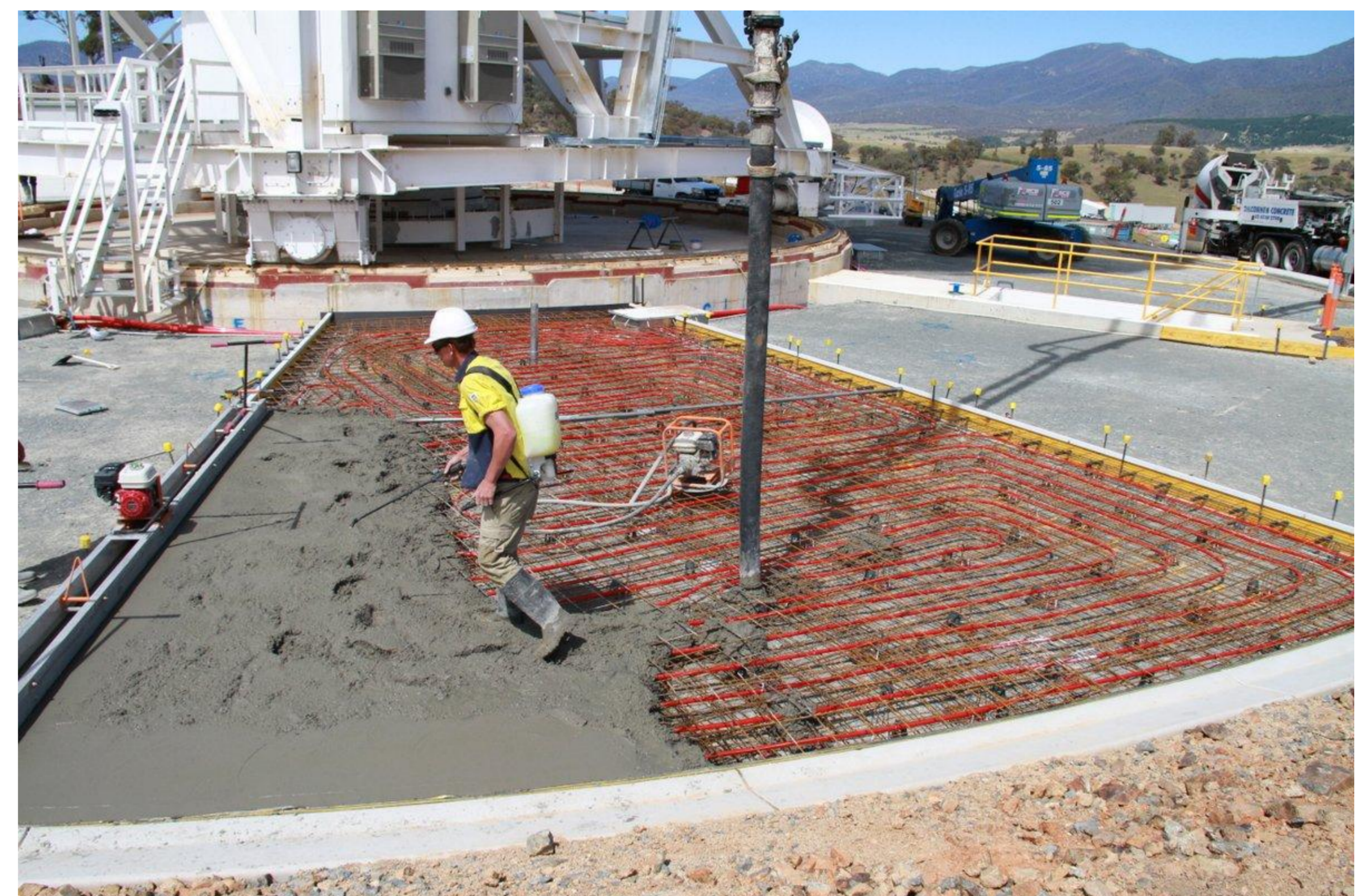
Figure 1: Installation of the night cooling system during construction of the antenna pedestal in November 2013. (Photo: Barry Davis)
