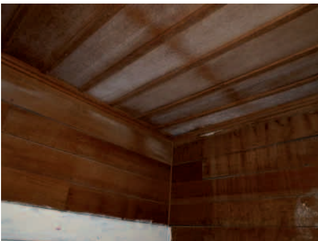
17 (top). Detail of the west elevation showing a fragment of timber at the north west corner of the roof suggested that there also had been decorative fretwork present.
