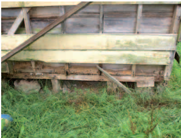
27 top). Detail of the main bearer after lifting of the building, showing the lap joint joining the two pieces of timber with puriri piles still attached.
