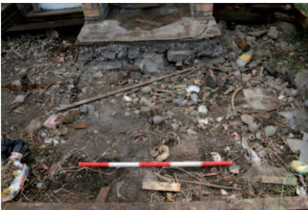
33 (bottom). The cottage footprint excavation in progress, showing the exposed fireplace and chimney foundation, bricks and rubble under the floor in the area around the back door, and scoria rubble under the floor of G3. Scales = 1 m.
