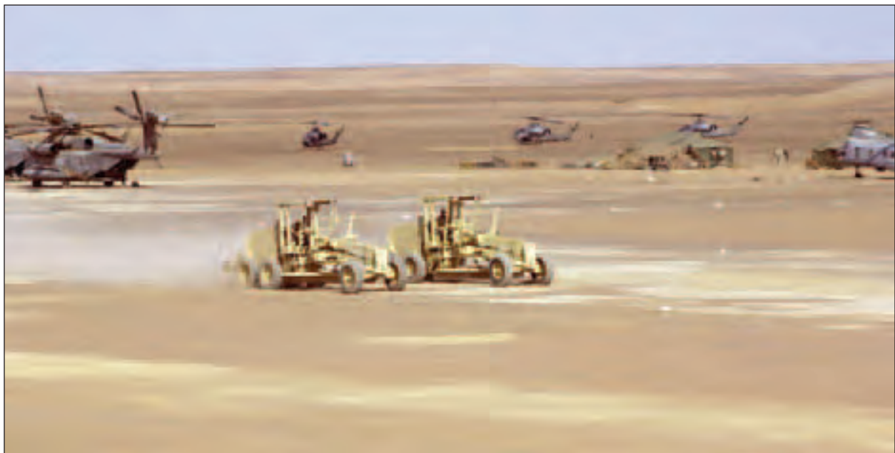
Seabees from Naval Mobile Construction Battalion 133 grade the runways at Camp Rhino, Afghanistan.
