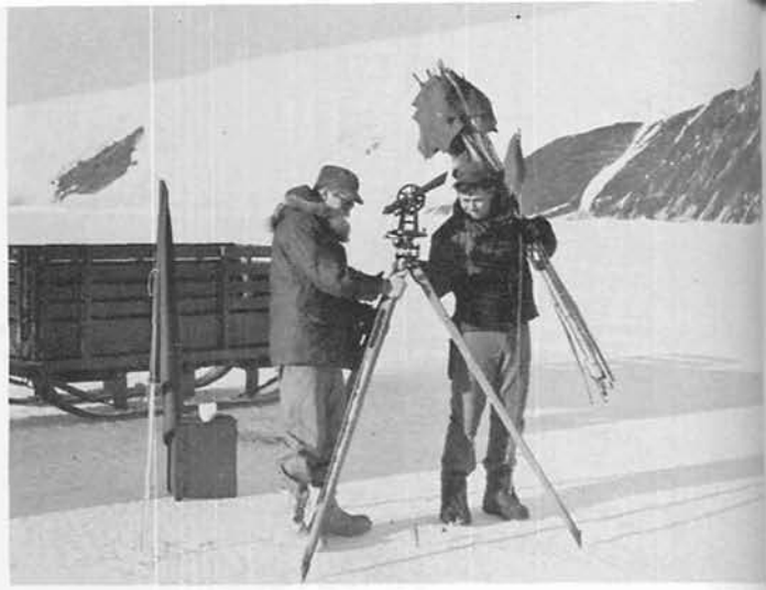
HALLETT'S Novasio and Hennessey set transit and stake markers during marking of emergency runway.
