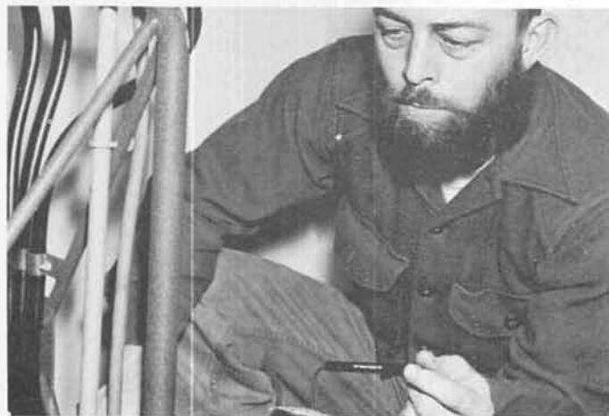
INSTALLING DF (direction-finding) equipment. Antenna is man-hauled to top of mast (above) in stiff breeze as Fred Charlton (below) wires receiver to pull in signals.
