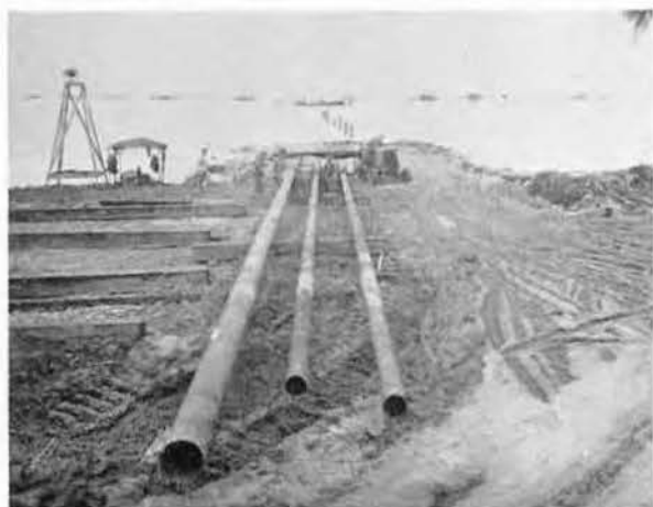
Fueling lines from the tank farm
