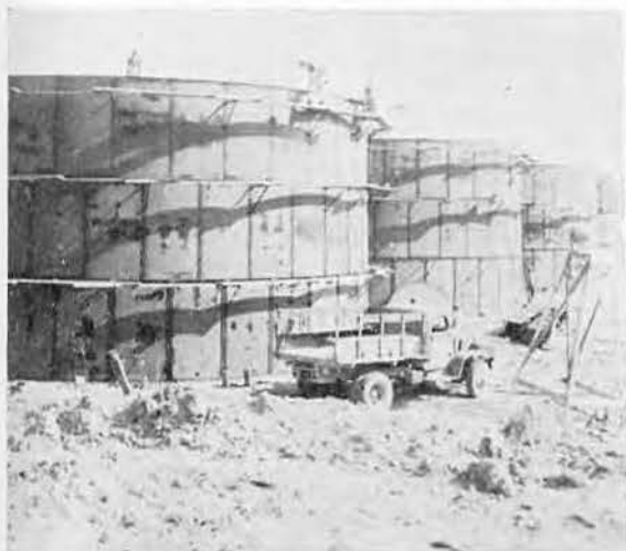
Friday . . . finishing touches are put on the tanks— and the Japs decided to call it a day too
