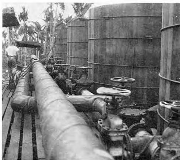
Water supply tanks and lines in Philippines
