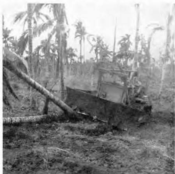
A bulldozer pushes over a couple of coconut trees in clearing operations
