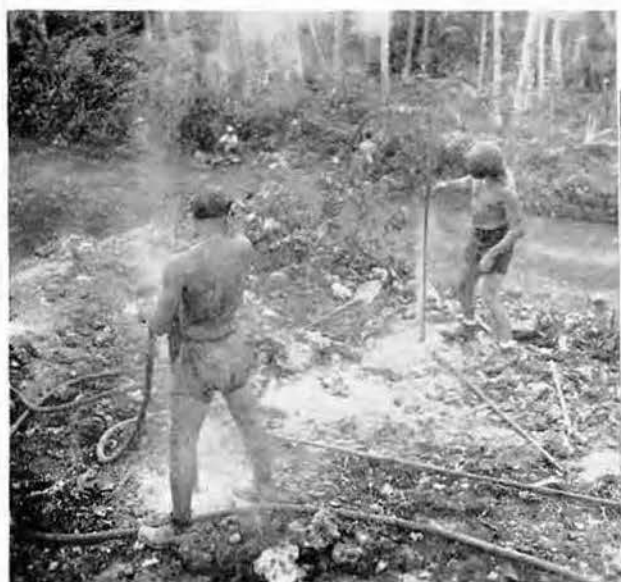
When the going is too tough, drillers and dynamiters are called in
