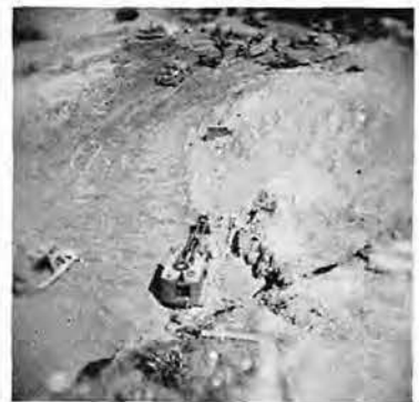
Gravel from this hill, near the point of our original landing, supplies fill for soupy roads
