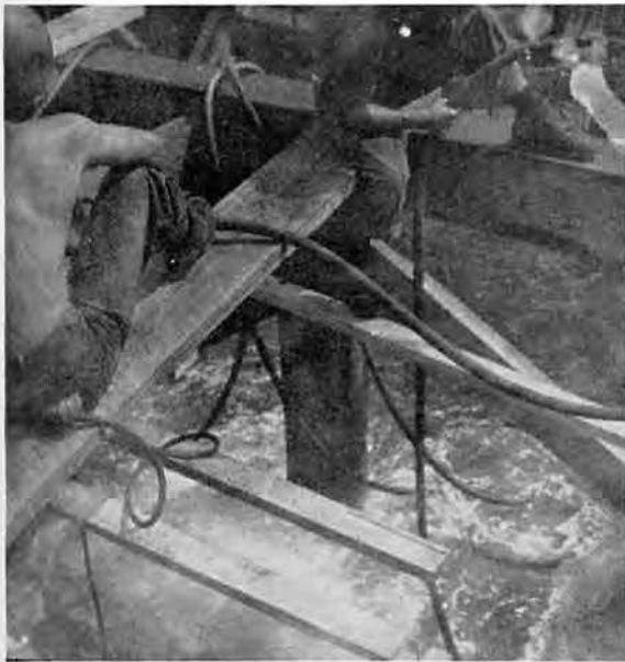
Bolting braces to piling under water is done by the diving crew
