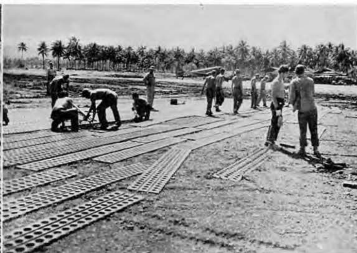
Marston matting has built strips from Guinea to the fringes of Tokyo. Here the 105th lays down part of its share
