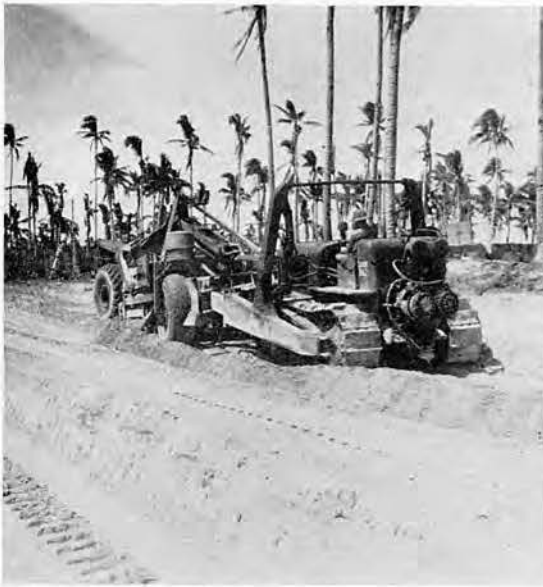
The road begins to take shape. A push cat loads a turnapull
