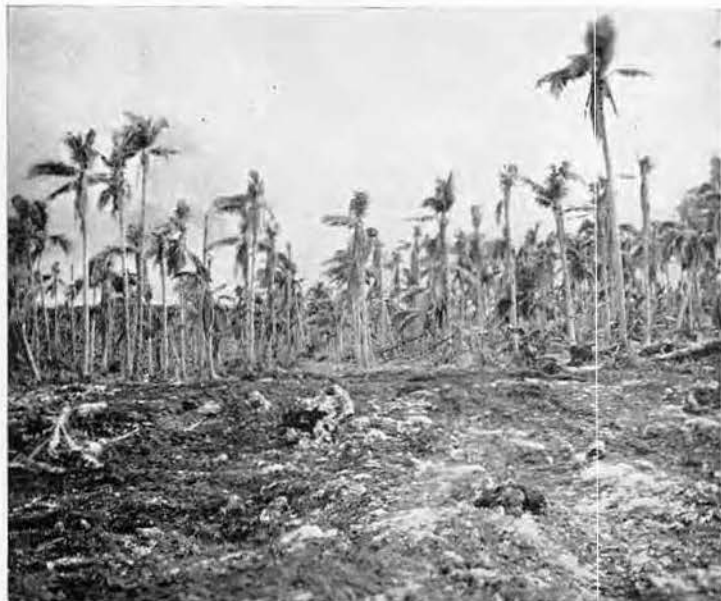
Carving roads through jungle, swamps and hills is an important and rugged job, requiring skill and knowledge
