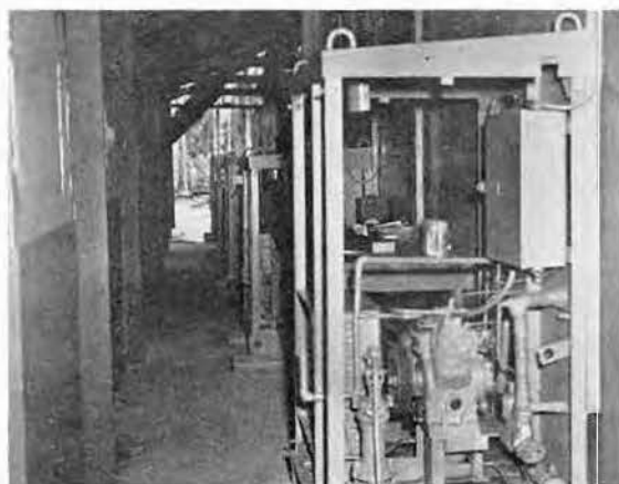
View of refrigeration units
