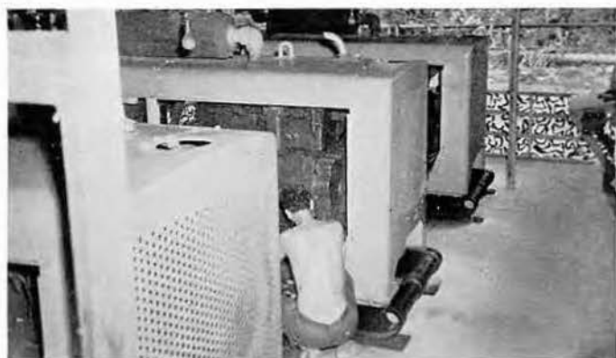
Generators which provide our light and power
