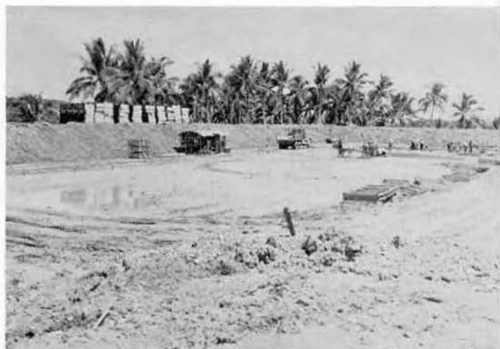
The tank farm—fuel and oil storage tanks—was our last job when the Japs threw up the sponge. On Monday the area looked like this
