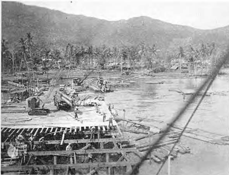
Where heavier docking facilities are required, the 105th tackles a job like this one in New Guinea
