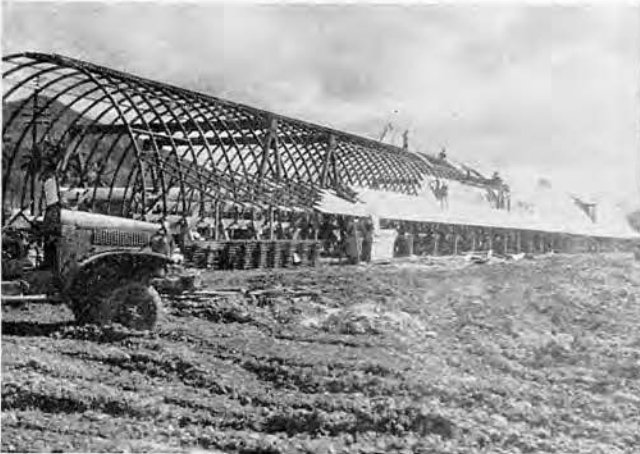
Ribs of this warehouse are in place and the roof is being rapidly completed
