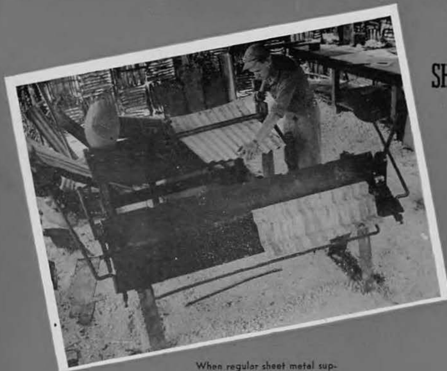
When regular sheet metal supply is low, corrugated quonset steel serves as a substitute with the metal workers.
