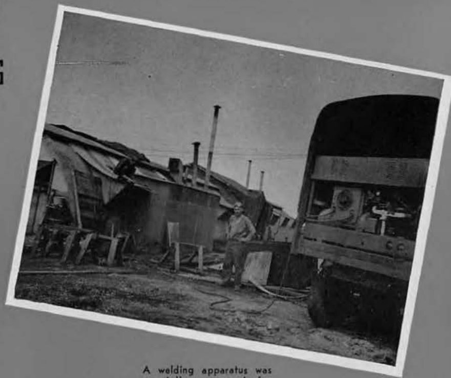
A welding apparatus was specially arranged for transportation on the job anywhere.
