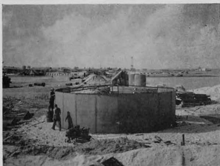
with tanks and pipe lines.
