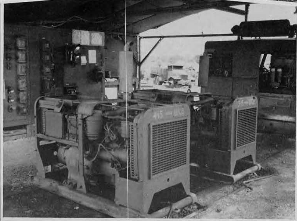
A generator power station.
