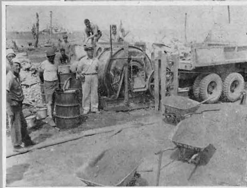
Right: A Jap cement mixer hitched to a truck was put into operation.
