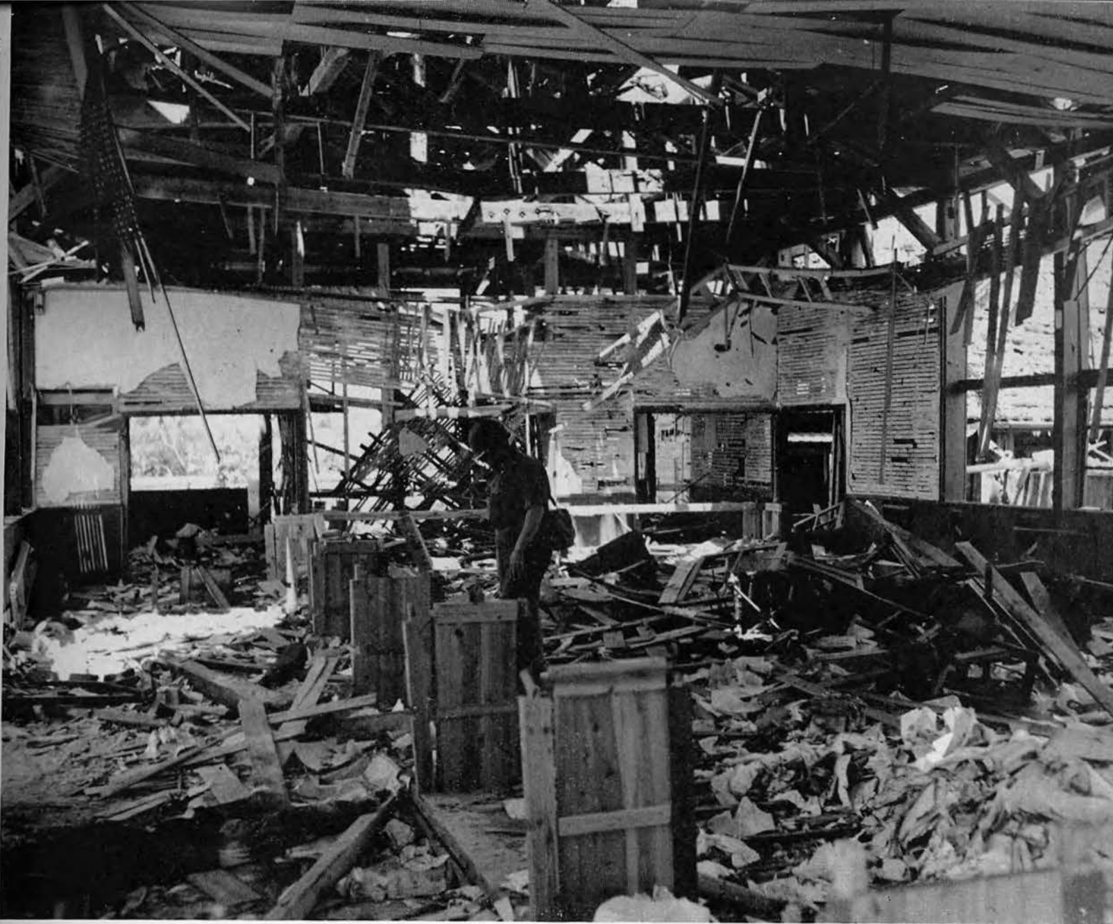
Wrecked City Hall
