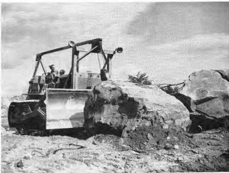
The Bulldozer Pushes Away Heavy Rocks Thus Clearing and Levelling a Roadbed.
