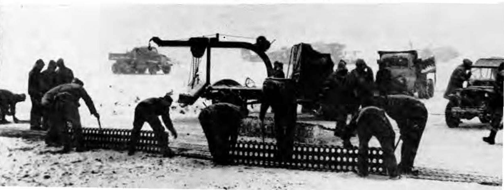
Seabees work through a williwaw (a mile-a-minute gale) laying marston mat at this Aleutian base, from which American planes took off to bomb Paramushiru, key Jap stronghold in the Kuriles.
