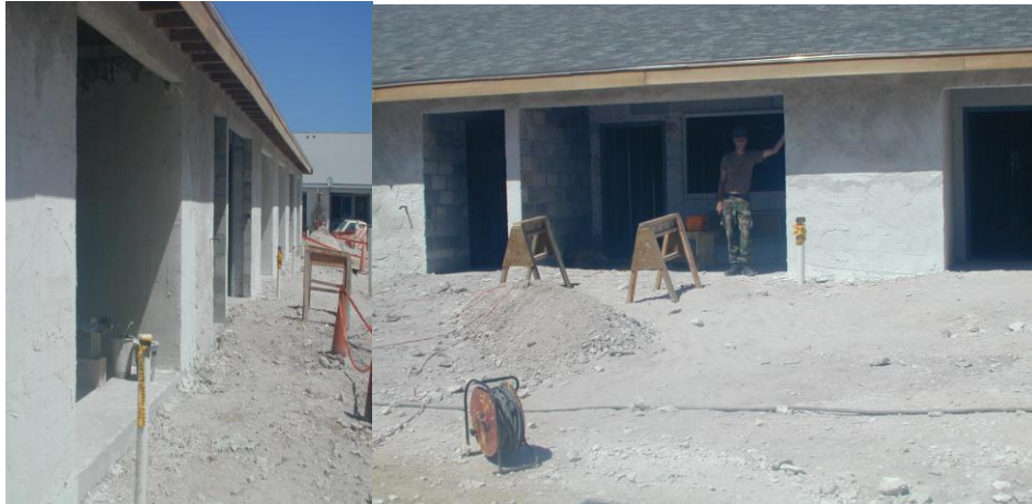
NMCB 26 and 21 personnel provided construction and management services support towards the construction of CBH 12 and 13 on Andros Island, Bahamas.
