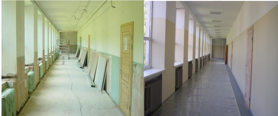
NMCB 26 renovated 80 lm of corridor & two stairwells in an Elementary school located in Tapa, Estonia. The project was performed under the auspices of the Partnership-for-Peace.
