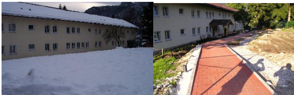
NMCB 26 provided a range of support at NATO's school in Oberammergau, Germany. Construction of handicapped ramps and a new facilities entrance (pictured above) are representative of the project.
