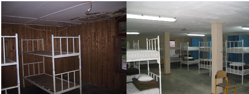
Barracks #8 before and after renovation – Seven detachments of NMCB TWO SIX personnel performed a full range of renovation services in support of Adriatic PHIBLEX 04, a multinational exercise held in Croatia.
