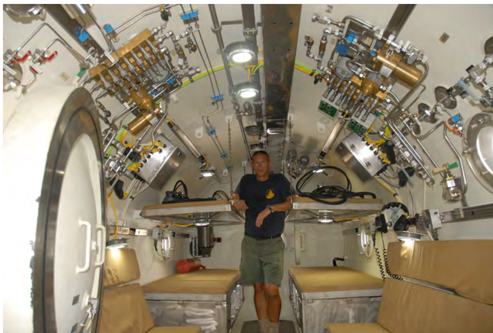
Figure 13-3. SAT FADS DDC Interior.
