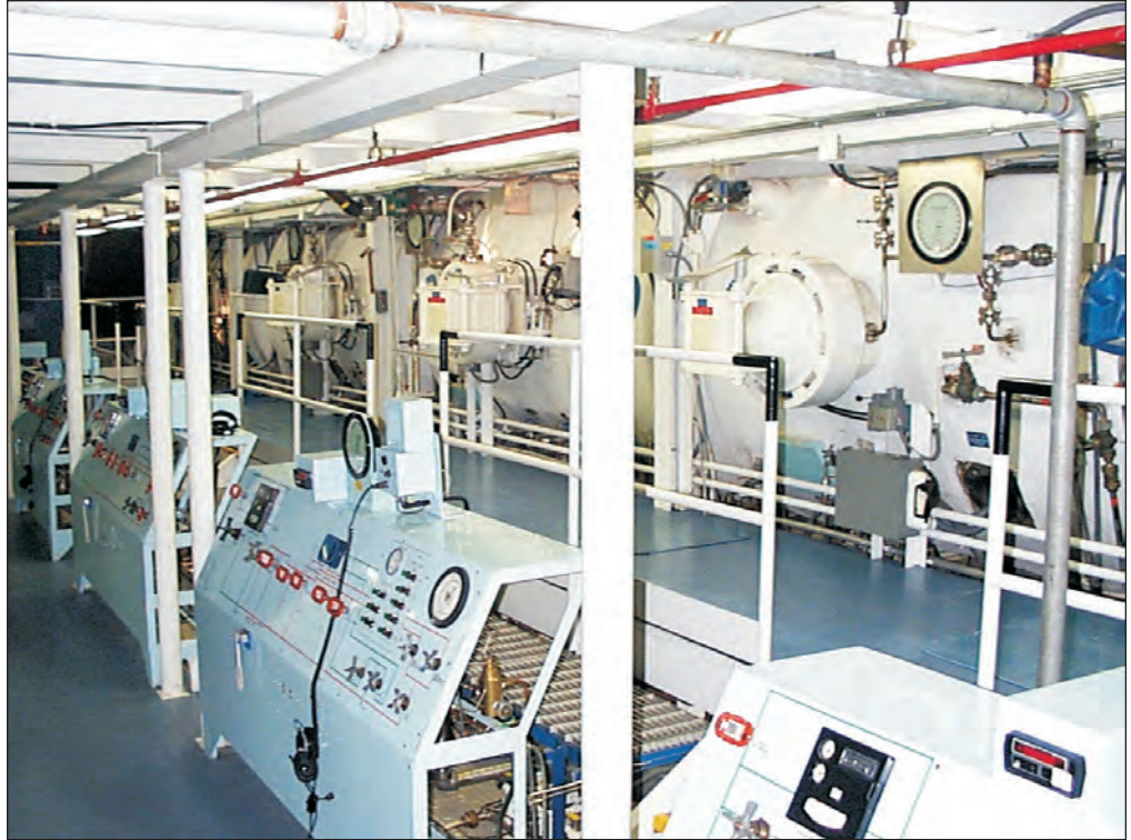
Figure 13-8. NEDU's Ocean Simulation Facility Saturation Diving Chamber Complex.
