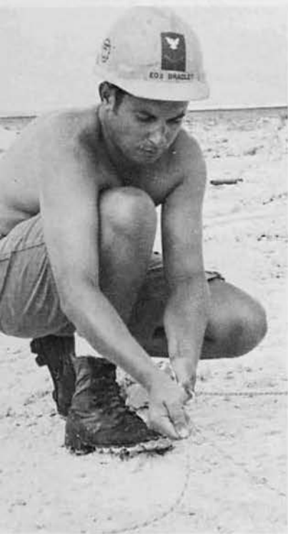
EO3 Ervin Bradley ties dynamite into det cord trunk lines preparatory to blasting.
