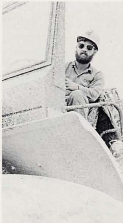
EO3 Bruce Baust operates an MRS scraper on the causeway. The MRS is an ungainly monster that was a real workhorse for A Co.
