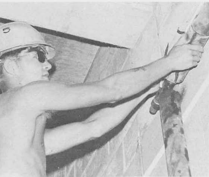
UTCN William "Oz" Osborne, Monsey, N. Y. , insulates an air conditioning line at the chapel.
