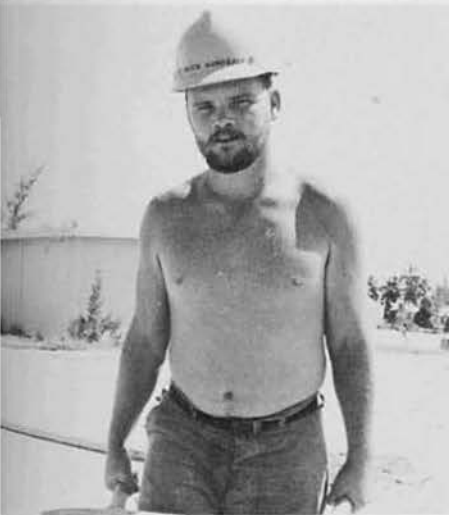
BUCN Carl "Nordy" Nordback, Stone Lake, Wis., carries fill to a curb and gutter site.
