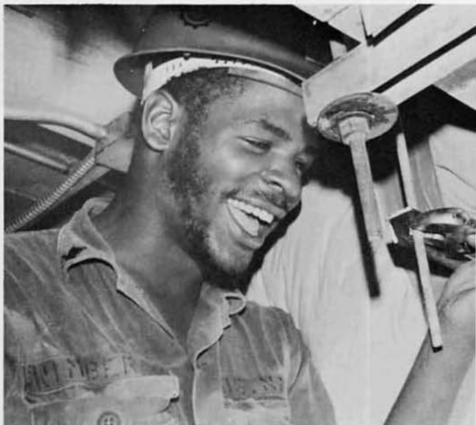
SW3 Richie Wimberley, Paterson, N.J., installs supports for air handling unit at the NEX.
