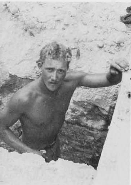
UT3 Doug "Babbitt" Beckwith, Babbitt, Minn., had a hand in installing the NEX sewer line.
