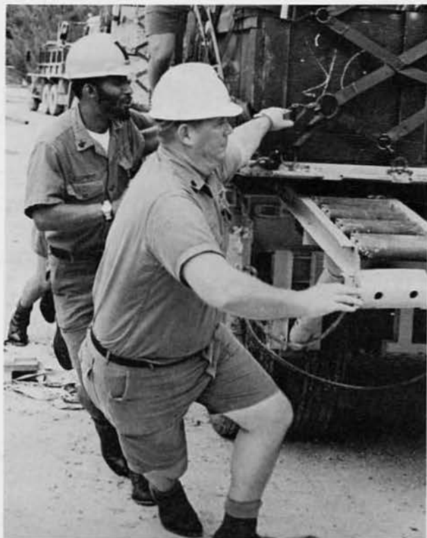
YN3 Archie Topps and BUC Robert Kemp, Silsbee, Texas, unload advance party gear. Chief Kemp was a projects supervisor.
