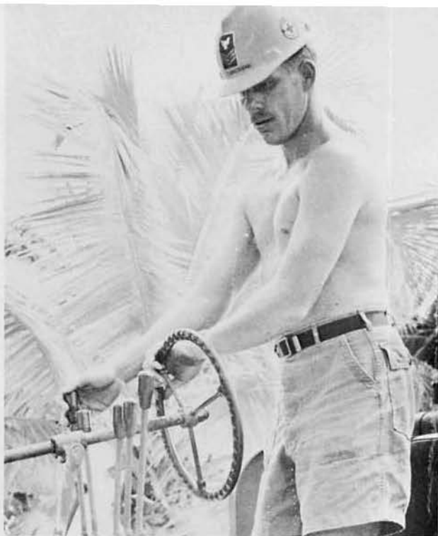
EO1 Steven Zimmerman grades a pad for the porta-heads in the camp area. Zimmerman was also yard boss for a spell.
