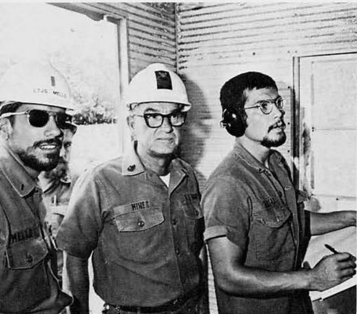
LTJG Raymond Mello, Fall River, Mass., BUC Robert Hines, St. Louis, Mich., and CE3 Al Arias take amperage readings at the MUSE emergency generator.
