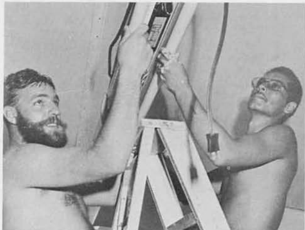
CE2 Sandy Sanderson and CE3 Ron "Mondegrove" Monreal, Ajo, Ariz., finish installing a new light fixture in the coffee house.
