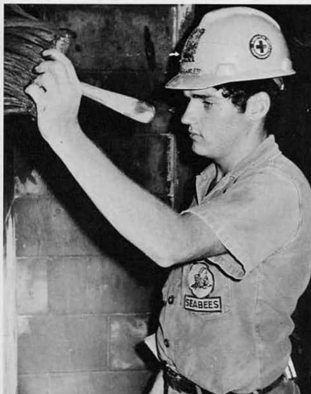
BU3 Dave Minkler, East Aurora, N. Y., applies "Slurry" coat (cement and water) to block wall prior to painting.
