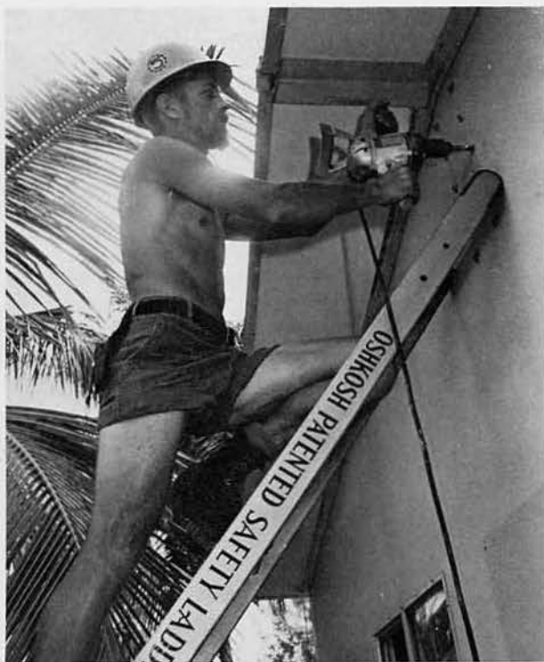
CE2 Tim Baird, Cass Lake, Minn., tightens anchor bolts for rehab wiring done at the coffee house-TV lounge.
