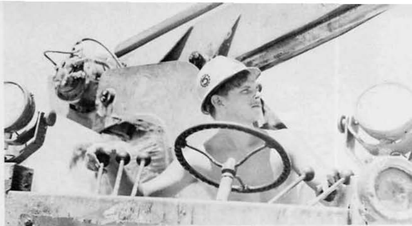
EO3 John "Watah" Powell, Boulder, Mont., uses the 10-ton cherry picker to literally raise the roof on a porta-hut.
