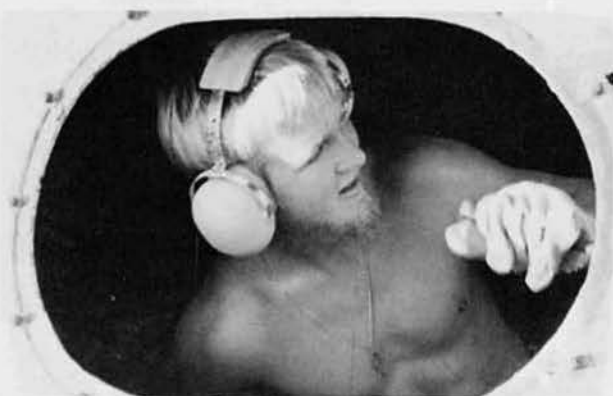
EOCA Paul Vornbrock chips the old family recipe from the inside of a transit mixer.
