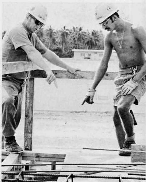
BU2 Don Underwood and BUCN Daryl Mackenthun, Allen Park, Mich. , discuss overhead forming placement.
