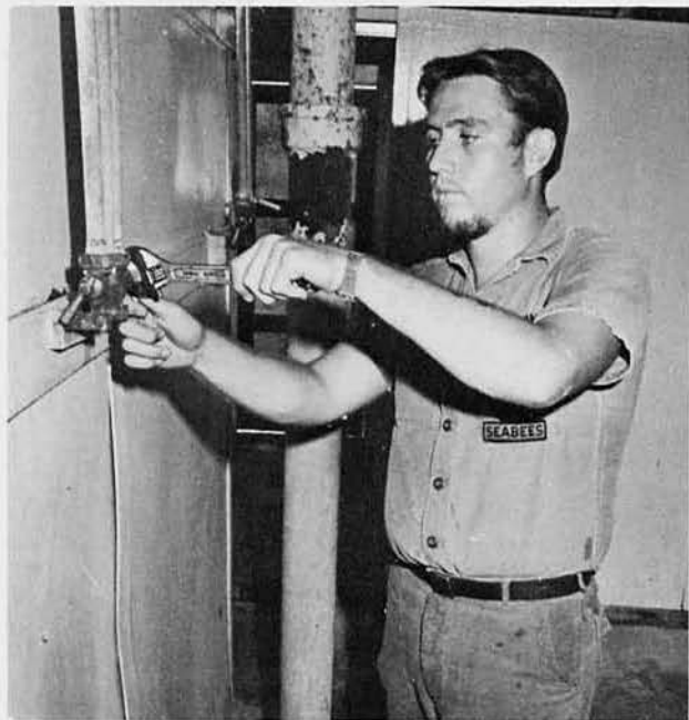
UTON Ed "Big Eddy" Tatro, Beloit, Wis. , repairs a shower in a camp head.
