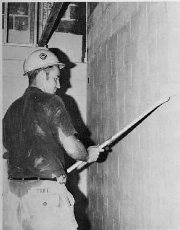
BU3 Rick Friel, Renovo, Pa., paints one of the NEX block walls.
