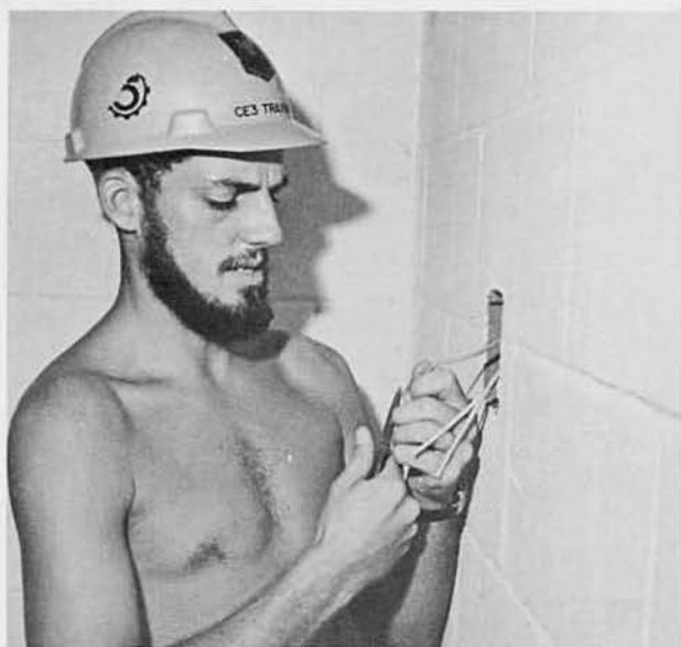
CE3 Steven "Trax" Traxinger, Minot, N.D., strips wires for a light switch in the chapel.
