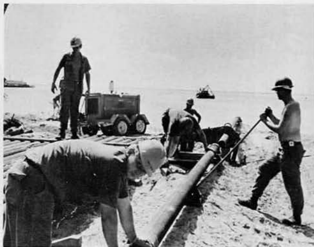
The temporary POL facility is the repository for the diesel fuel, MOGAS, and jet fuel used in island operations. Echo Co. steelworkers assembled 5,000 feet of six-inch pipe for use in off-loading.
