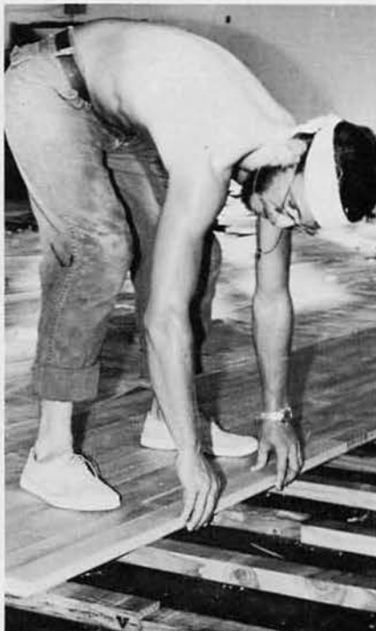
BU3 Willie Wetmore lines up floorboards for the hammer. The boards were tongue and groove.
