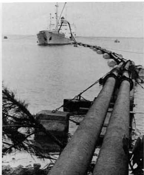
The concrete silos are loaded by blowing the cement from the cement ship through pipeline to the top of the silos.
