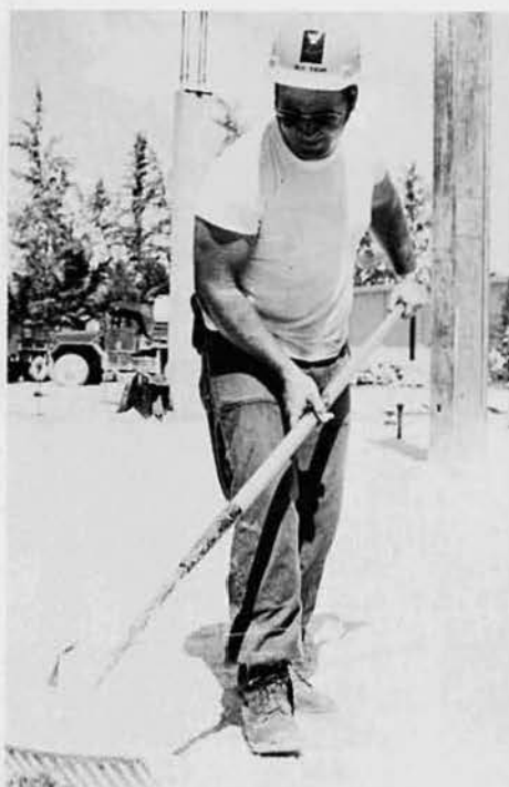
BU2 Vic Eagan, Newport, Ore., levels the pad for a concrete slab pour.
