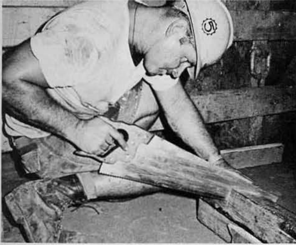
BU2 Earl "E. J." Copeland cuts dunnage during the January ship off-load. He was the curb and gutter crew leader.
