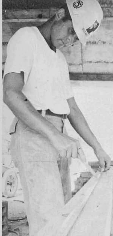
BU3 Dave Maez measures off lumber for formwork for the subsistence building.
