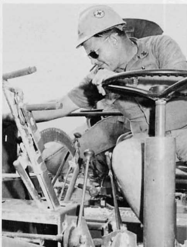
EO2 Tom Solbeck on the chip spreader, which lays an even layer of aggregate along the roadbeds.
