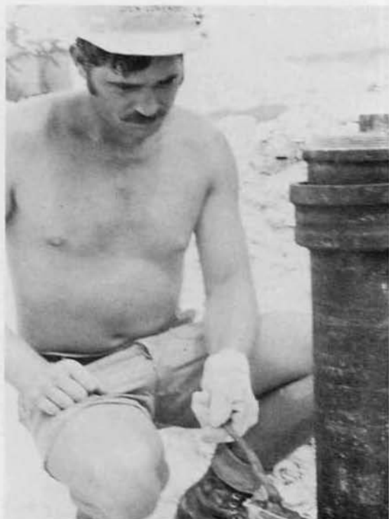
UTCN Ron Longworth, Columbus, Ohio, pours hot lead to a pipe joint at the subsistence building.
