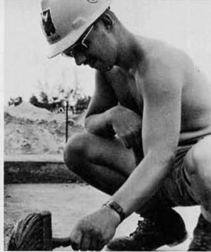
BU3 Robert Siuda, Palos Heights, Ill., does finish work on a dumpster pad.
