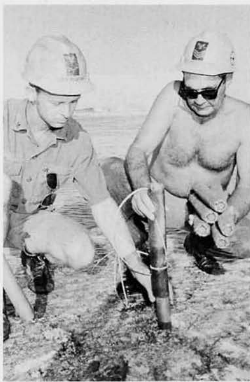
EO3 John "John Boy" Fulford and EO1 Owen Westberry load dynamite into the holes. One of the side effects of working with dynamite is a splitting headache, which tide haul learned to live with.
