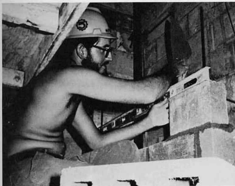
BU3 Tom "Moose" Mossman checks the level of block being laid in the shower rooms.
