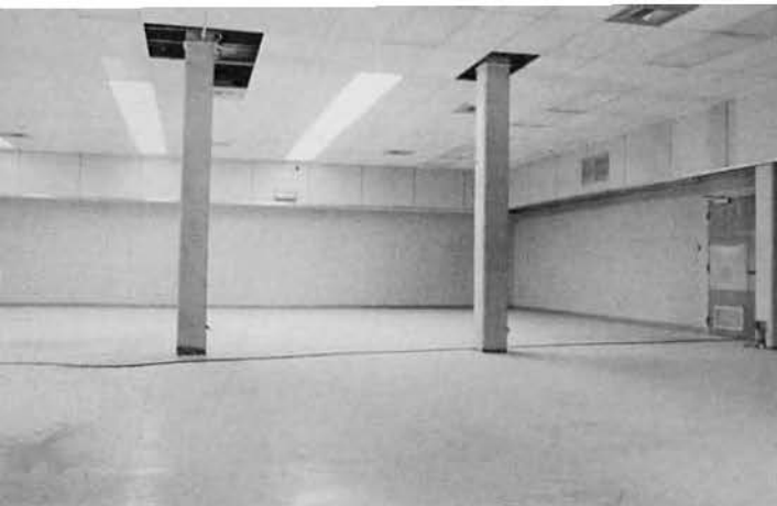
The main room of the Navy Exchange as it nears completion. The building was taken from 17 per cent to virtual completion by the 'Bees of FIVE.
