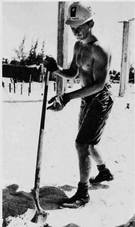
BU2 Chris Rauch, Oxnard, Ca., works sub-base material at the subsistence building.
