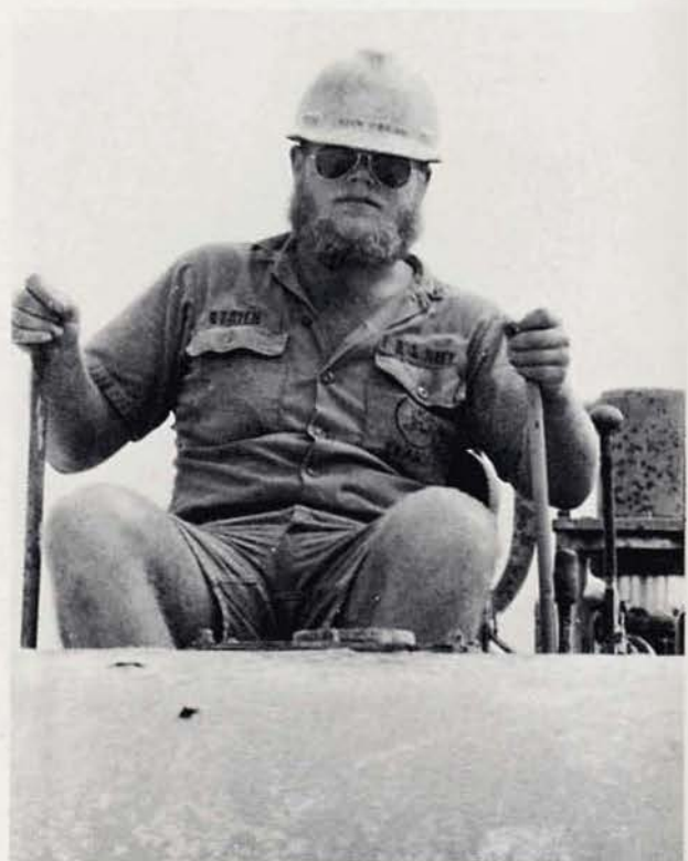
EOCN Michael "the Mangy Dog" O'Brien operates a roller on the causeway, preparing it for paving.
