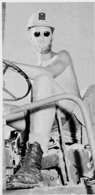
EOCN Dwight Mahaffy, Inglewood, Calif., hauled coral to the rock crusher in an MRS (Mississippi Road Service) side dump.
