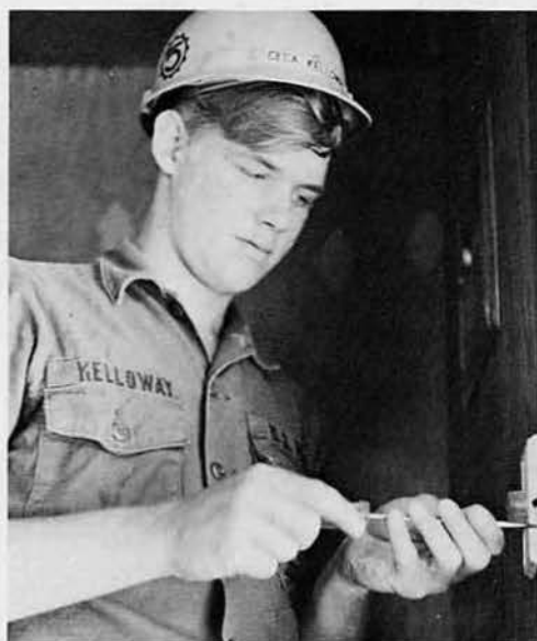
TOP LEFT: CECA William "Scamp" Scampoli, Bronx, N. Y., puts a loop in a guy wire. TOP RIGHT: CECN George Weatherford, Holly Springs, Miss., digs a trench between the exchange and the sub building. RIGHT: CECA Joel Kelloway, Nashua, N. H. installs a rheostat in a porta-hut.
