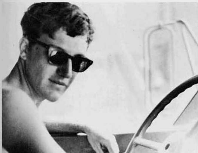
EOCA Randy Granger, Thompson, Ohio, hauls asphalt to the POL via 5-ton dump.
