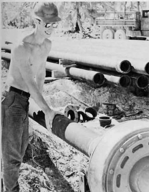
SWCA Richard Garrett, Wheatland, Mo., fits a pipe into the power tong at the temporary POL facility.
