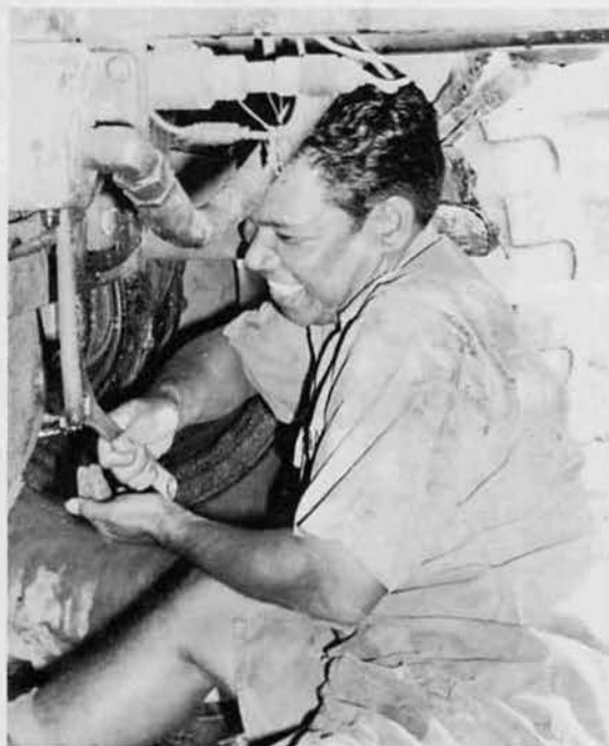
CM2 Jose Cruz checks differential lubricant at the heavy shop lube shop. LEFT: CMCN Rick "Jake" Jacobsen, Portland, Ore., works on a boom lift ram hydraulic hose on a Hough 120.
