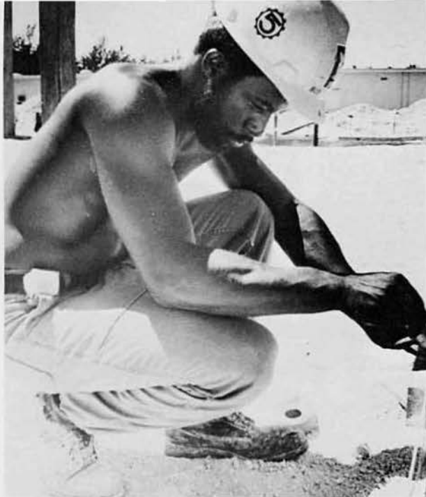
BU3 David "Good Old Norm" Norman, Yonkers, N. Y., puts batter-boards in at the subsistence building.
