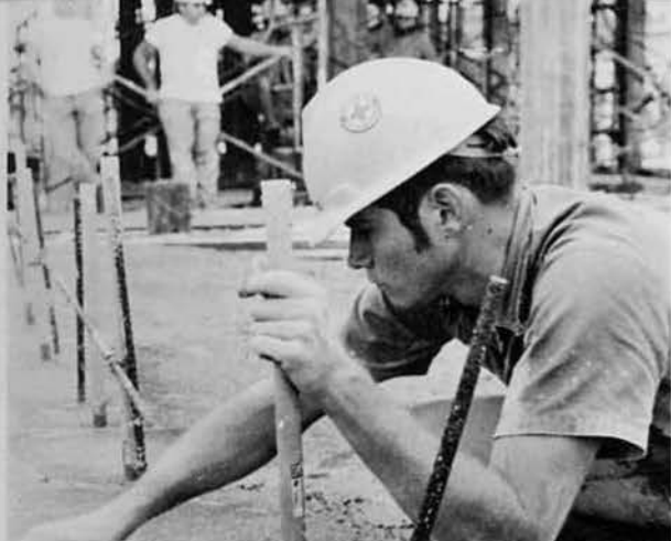
BU3 George Monroe, Arvada, Colo., finishes a concrete slab on the subsistence building.
