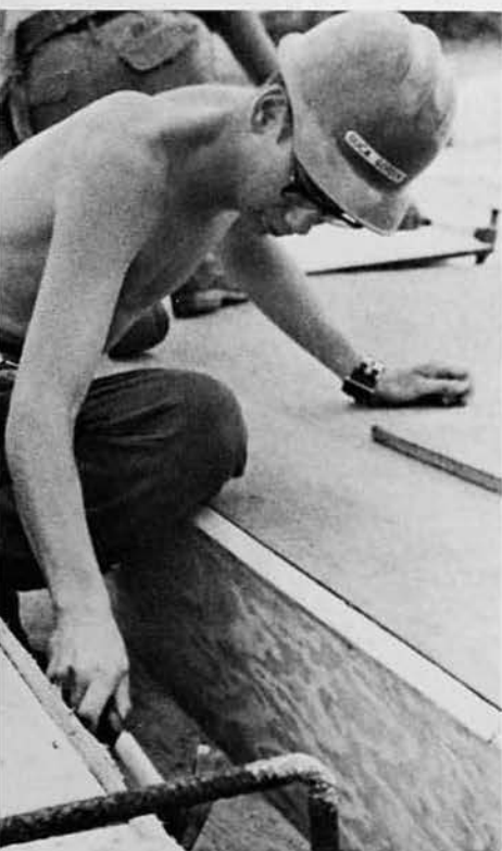
BUCA Charles Gordon, Ballston Lake, N. Y. , nails in chamfer strip in an overhead bond beam.
