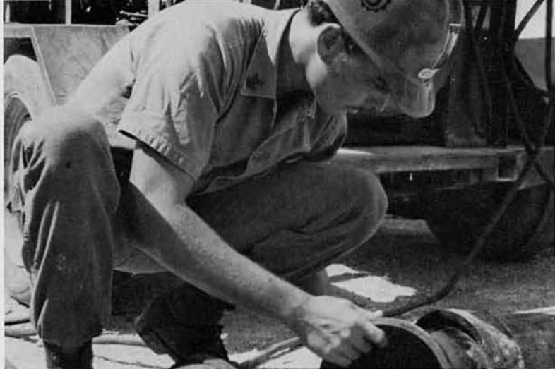
UT2 Billy R. Haley, Dearborn Heights, Mich., fits an elbow to a straight pipe for a camp sewer line improvement.
