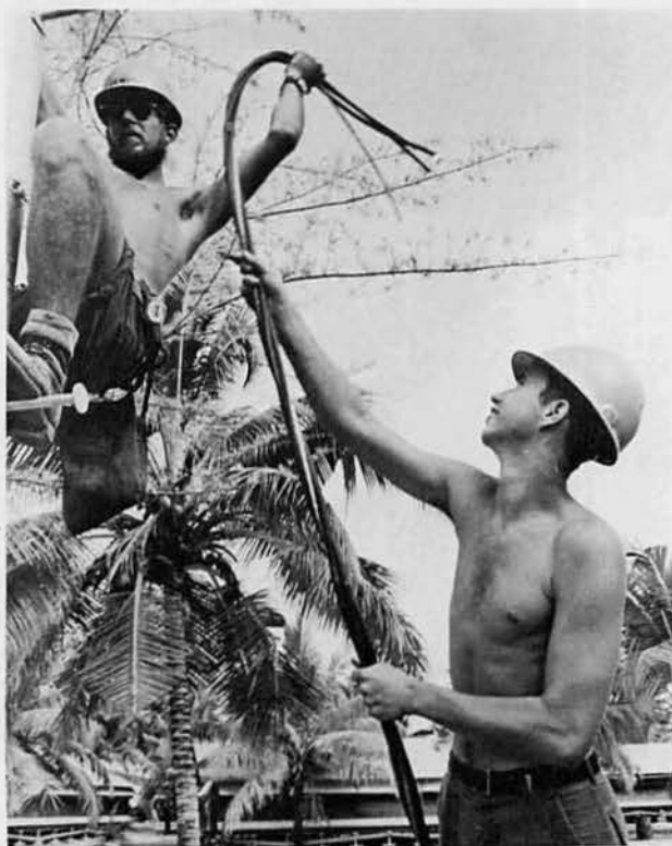
CECA Robert "Newt" Newton, Ojai, Ca., and CECA John "Cookie" Cook run new power line in the camp area.
