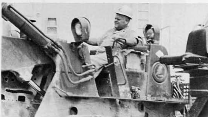
EO3 Wally Chappell backfills a utility trench at the subsistence building with a 175 IH back-hoe/front end loader.
