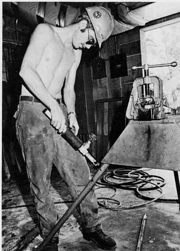
UTCN Alan "Zobe" Zobel, Roosevelt, Utah, also works on chapel air conditioning line insulation.
