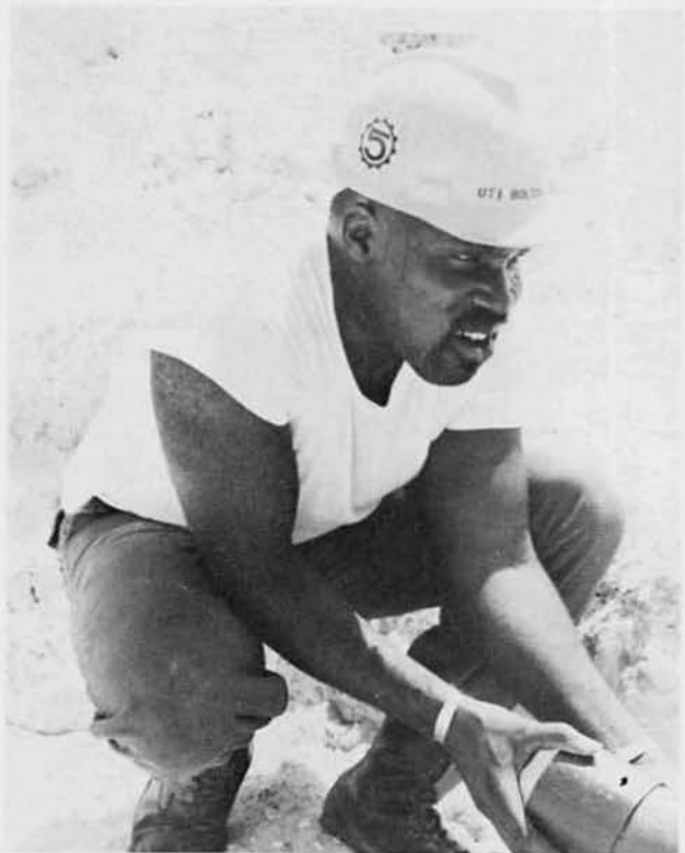
UT1 Cal Bolton, Atlanta, Ga., puts a coupling on pipe at a porta-head, where he was a crew supervisor.
