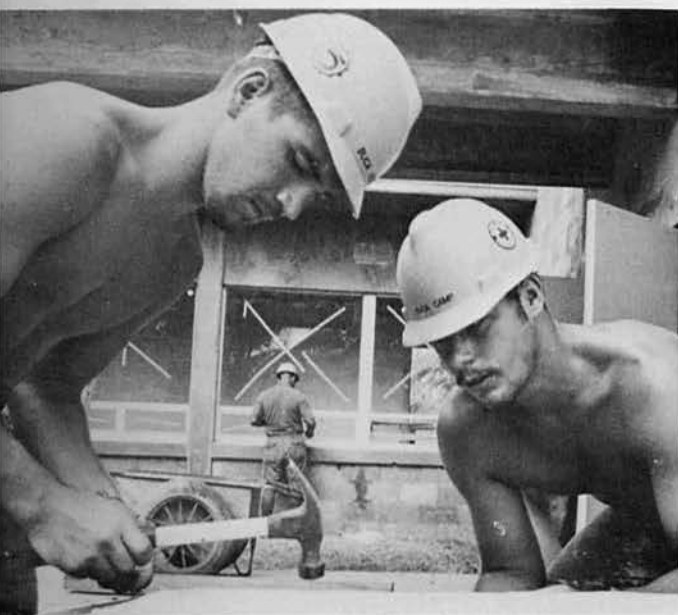
BUCN Dennis "Buffalo" Hebert, Newport, Vt., and BUCA Neal Camp, Merced, Ca., repair a door at the chapel.
