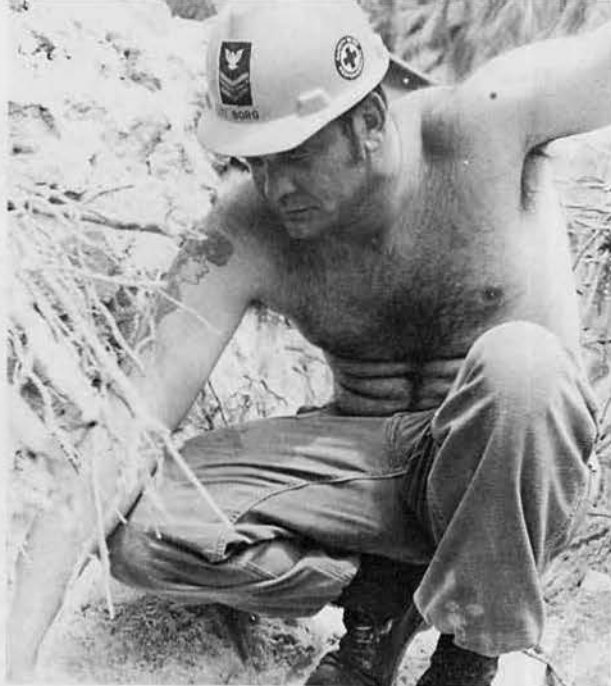
UT1 Dave Borg checks his crew's work on a storm sewer at the Navy exchange.
