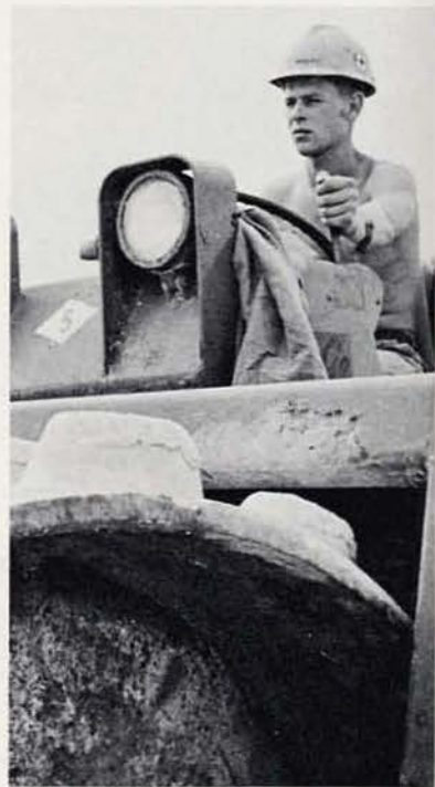
EOCA Scott Magley compacts the POL causeway with a RayCo roller. The entire POL crew put in many long hours completing the job.
