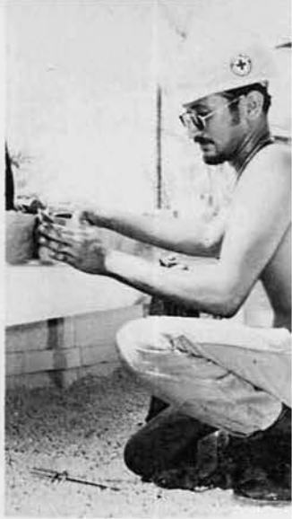
BUCN Rich "Black Bean" Yrigollen, Madera, Ca., tapes gravel stop around the top of the chapel.
