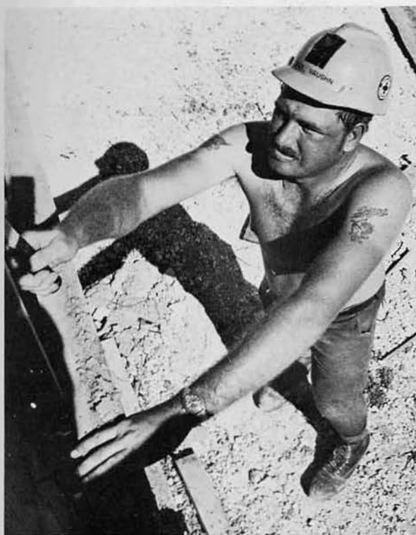
BU3 Jimmie Vaughn, Benton, Ky., nails walers (side braces) into place at the incinerator.
