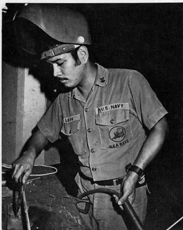
SW2 Lawrence Leonguerrero, San Jose, Ca., does a simple weld in the steel-worker shop. LEFT: SWCN Tom Pharo on the reefer warehouse rehab job.
