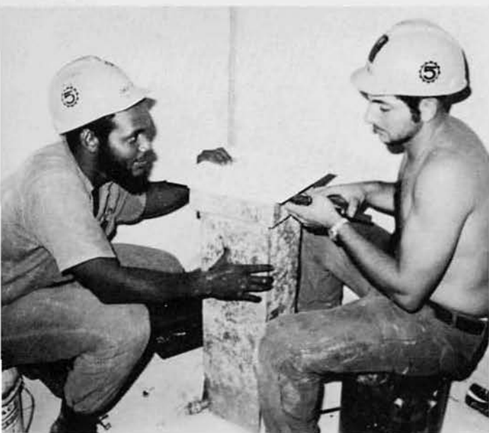
SWCN Clarence Love, Kansas City, Kansas, and SW3 James Bill, Bay City, Mich., fabricate duct work at the chapel. Love was Seabee of the Month for March.
