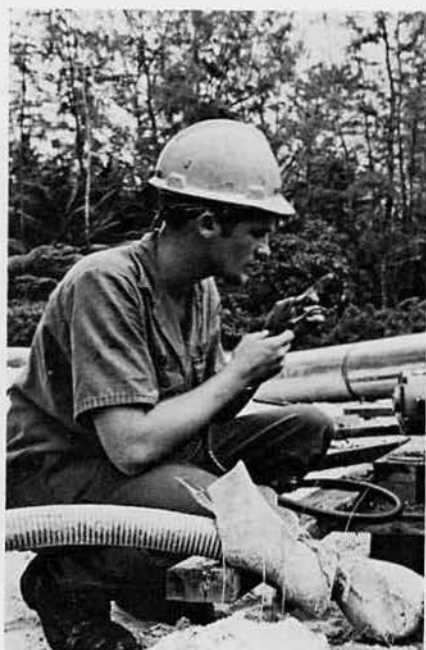
UTCN Frank "Skip" Baird hooks up a pump at a well site. Rehabbing and improving the wells was one of FIVE's major projects.
