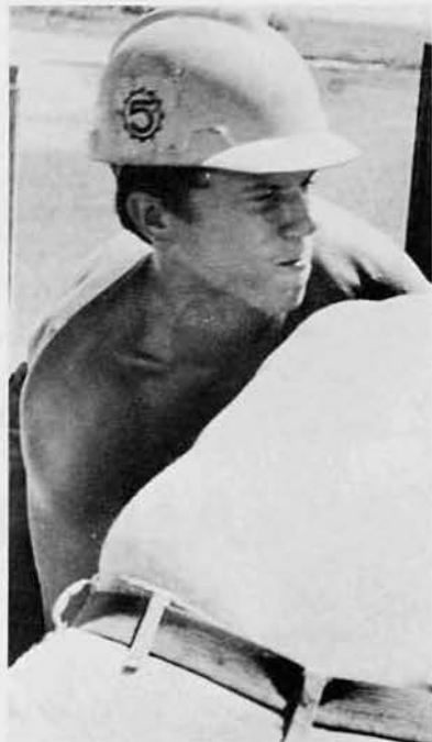
EOCA Clint Arrowwood, Corona, Calif., empties RC-250 asphalt into the melting pots. As with most of the Seabee jobs, a strong back is needed.
