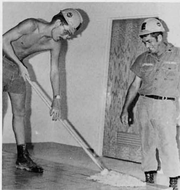
BU3 Jay Cannon, Costa Mesa, Ca., mops altar base in the chapel as BU2 Ed "Stinky" McCracken, project supervisor, observes.
