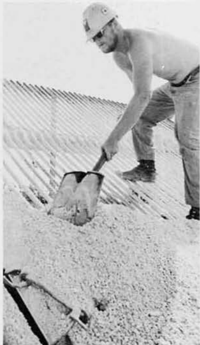
EO3 Ralph Felter, Sidney, N.Y., clears the screen over the aggregate bins. Ralph also worked on the POL and operated the crane during the ship off-load.
