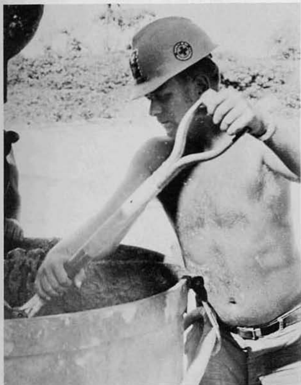
BU3 Don "Pooh-Bear" Russell, Fresno, Ca., shovels the concrete bucket clean at the incinerator.
