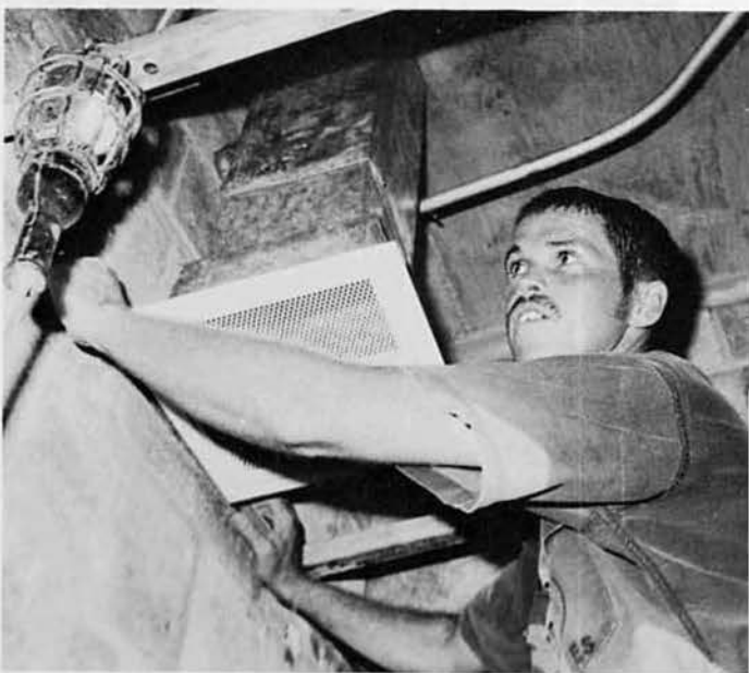
BU3 Dennis Hamilton, Portland, Ore., puts in a vent in the chapel drop ceiling.
