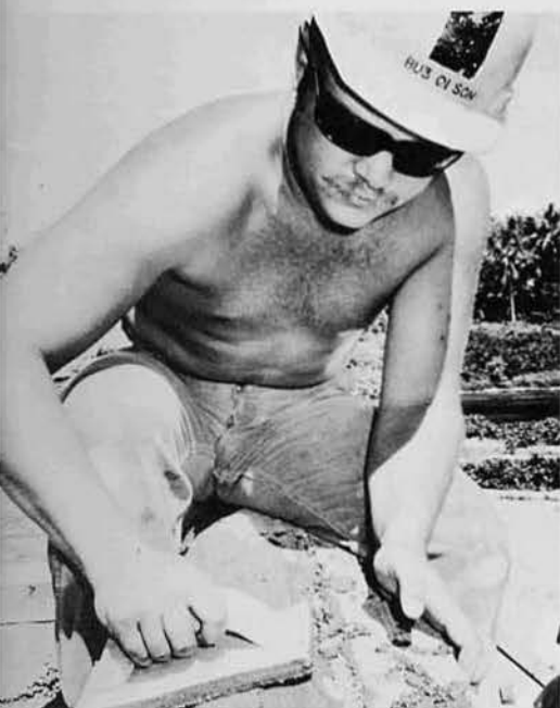
LEFT: BU3 Greg Olson finishes concrete at the incinerator. RIGHT: BUCN Tony Wright, Detroit, Mich., also helped erect the first porta-huts.
