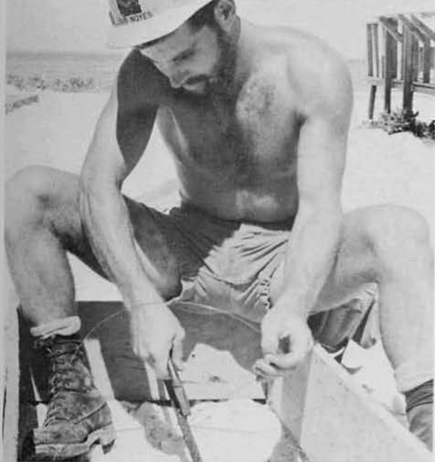
BU3 Alfred "Freddie" Noyes, Roseburg, Ore., uses tie wire to set formwork to correct width.
