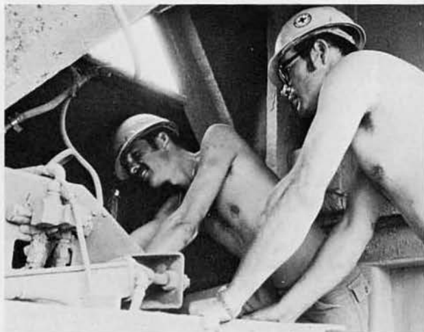
BUCN John "Dutch" Hamilton, Palm Springs, Ca., and EO1 Dennis Wooley at the concrete batch plant.
