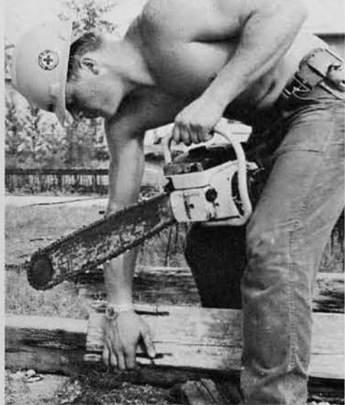
LEFT: BUCA Francis Sanker, Altona, Pa., cuts timber for a roof support beam.
