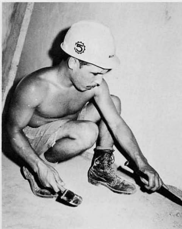
BUCA Jim Hunter, Quincy, Ca., cleans out expansion joints in the chapel.
