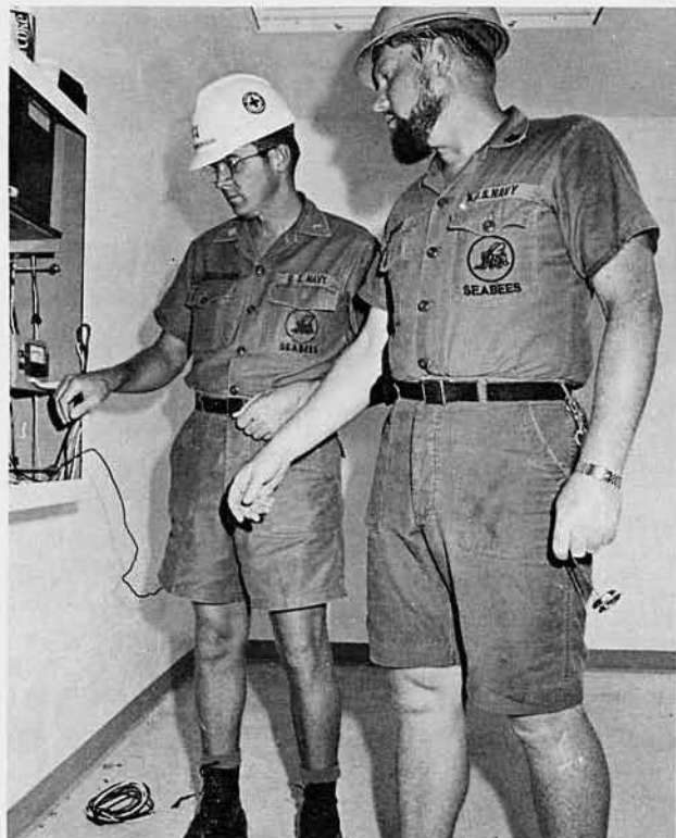
LT William Scarborough and CE1 William Bridges check Bravo Company CE work on the main relay panel in the sick bay operating room. LT Scarborough moved to the Training Officer slot in preparation for homeport.
