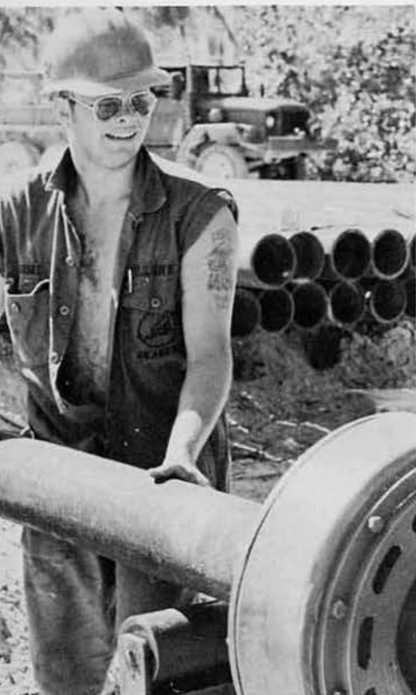
SWCN Ricky Barnes, Independence, Kansas, guides pipe into a power tong at the temporary POL.
