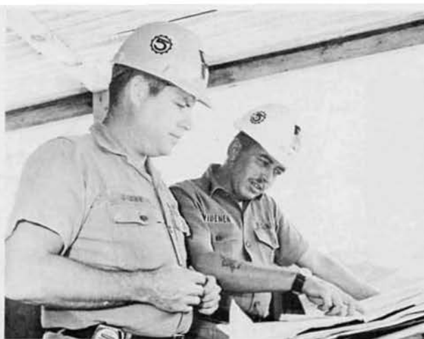
UT1 Robert Conway, Kansas City, Mo., and UTC Gary Widener read blueprints for water line at the subsistence building.
