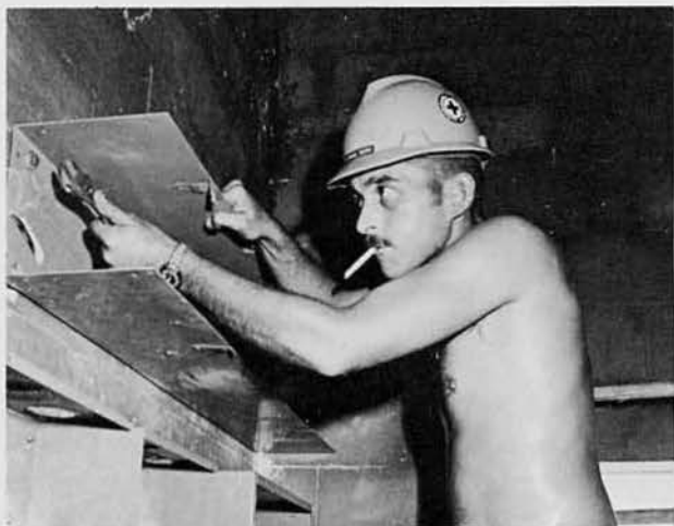
CE3 Larry Pival bolts a wire gutter over the power panels in the NEX.
