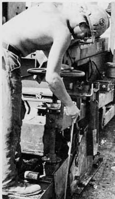
EOCN Bob "Lappod" Leppanen checks the thickness of the finished asphalt mat. Rollers will finish the job.
