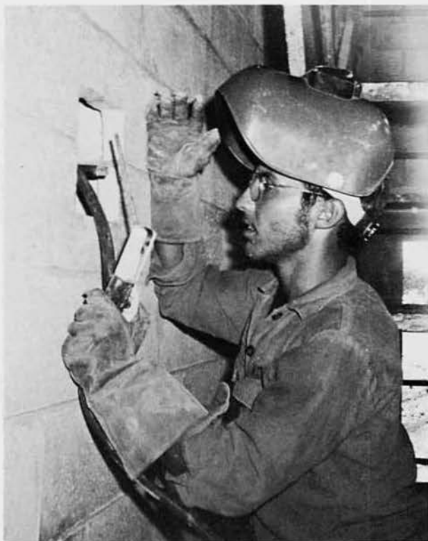
SWCN Phil Latronica welds a window winch into place at the gymnasium.
