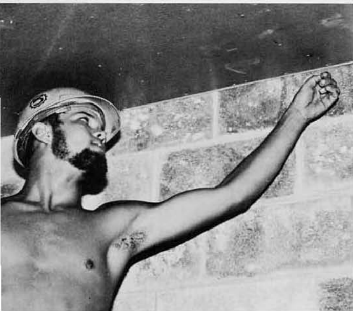
BUCN Ralph "Swamp-rat" Farr, Waycross, Ga., nails the ceiling in at the I-level maintenance building.
