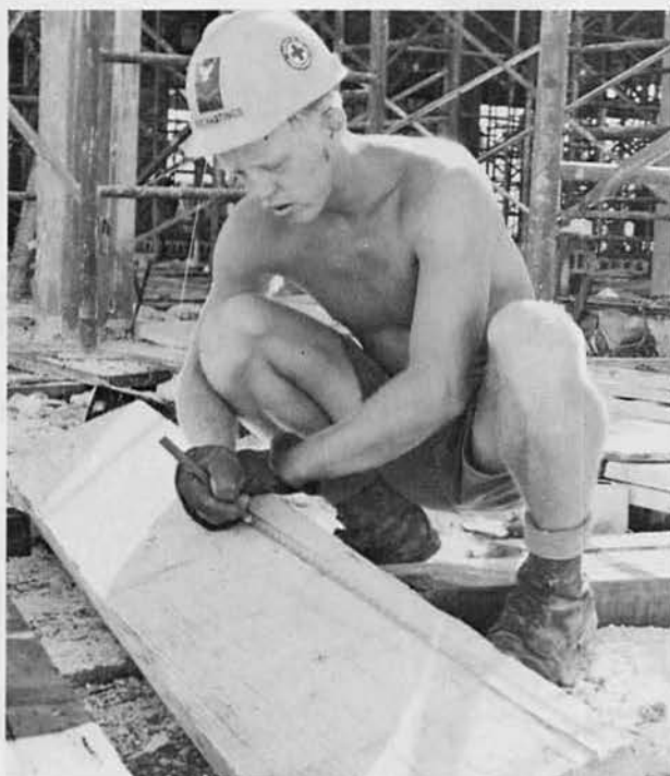
BU3 Bill Hastings, of the subsistence building forming crew, measures a beam for overhead formwork.
