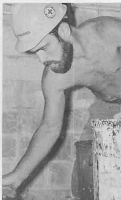
BUCN Mark Wyngarden, Madras, Ore., does patchwork on block walls. Mark is an avid bowler.
