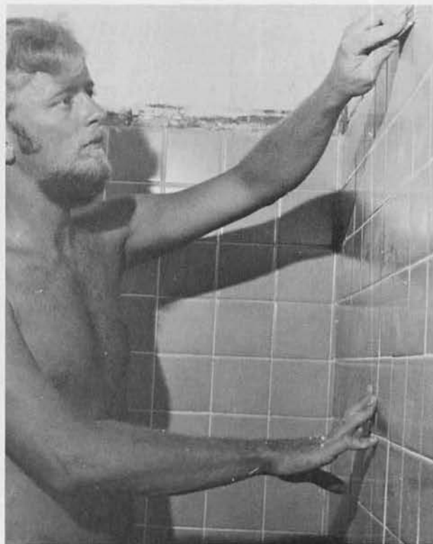
BU3 Walt Mistler, Portland, Ore., prepares the gymnasium shower room tile for upper molding.
