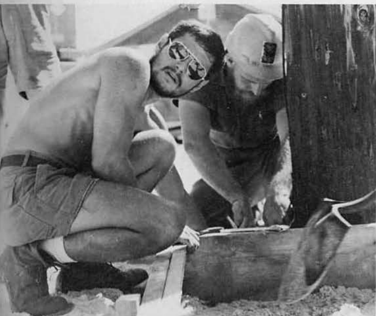
CE3 Al Arias and CE2 Johnny "Sandy" Sanderson place a grounding line for a transformer for the Camp Cummins electrical distribution system.
