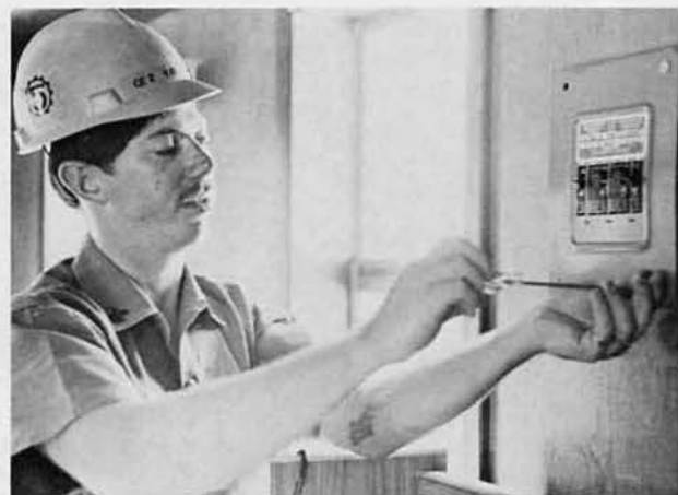
CE2 Art Violanti, Riverside, Ca., replaces the cover to a breaker box in one of the new porta-huts.
