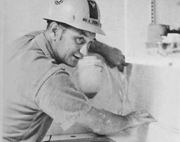
BU1 Jim Fowler, North Franklin, Conn., checks punchlist finish work at the medical facility. "Holy Catfish!"
