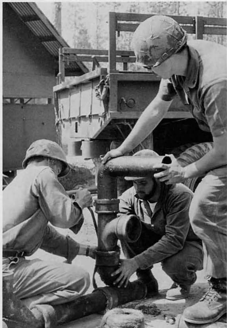
UT's connect a pipe as part of their plumbing project at Camp Swampy.
