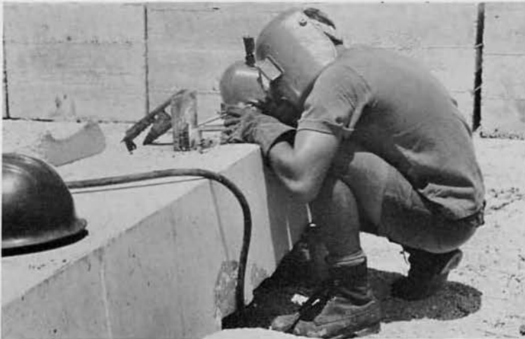
A steelworker welds a lifting eye on a power pole in the C Co. yard.
