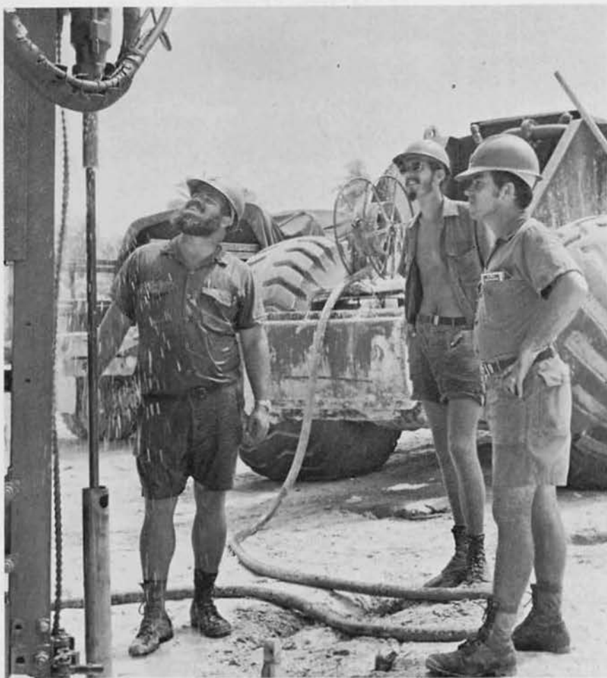
Ivey, Grajewski and Duke drill holes for dynamite charges at the wet well
