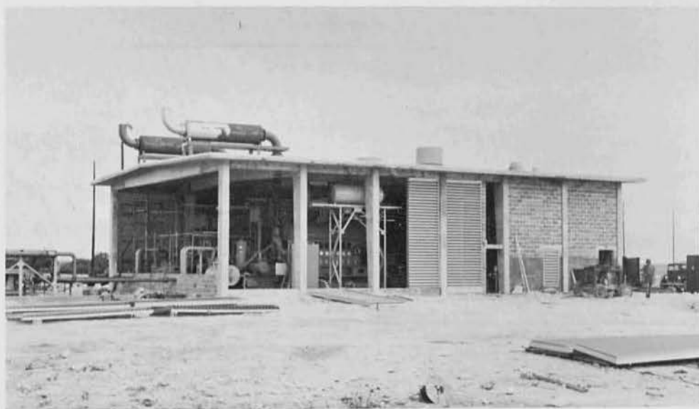
Standby Power #1 — placed on line by Sixty-Two
