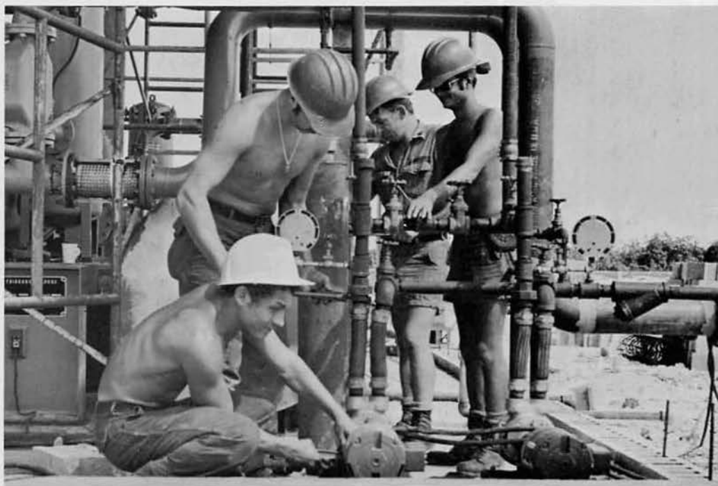
Standby Power 1 — a challenge successfully met by Bravo Co.
