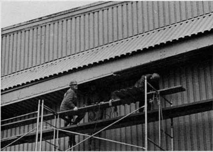
SW3 Cool, SW1 Ford, SW2 Van Overmeiren installing soffit on front overhang.
