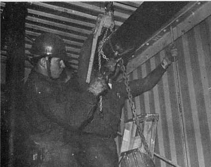
UT2 Fountain and UT2 Lewis installing trunk line on fire protection system.
