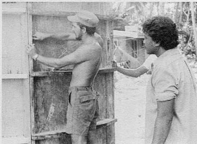
Marlow Draper and trainees bolt together forms for the Udot water tank.
