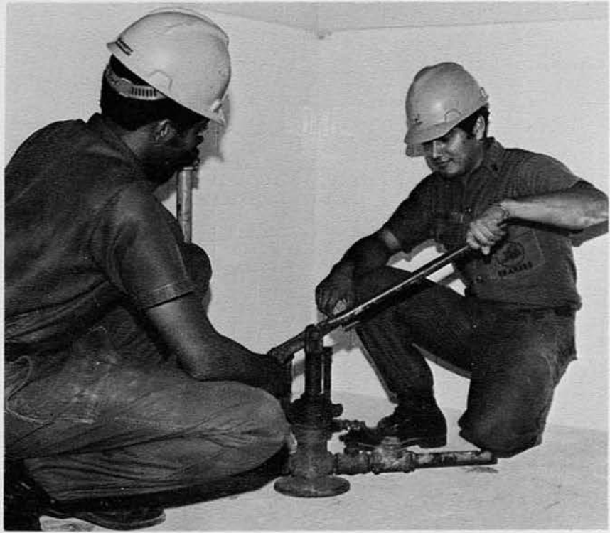
UT3 Telles and UTCN Willett preparing for hydroststic test of water piping system.
