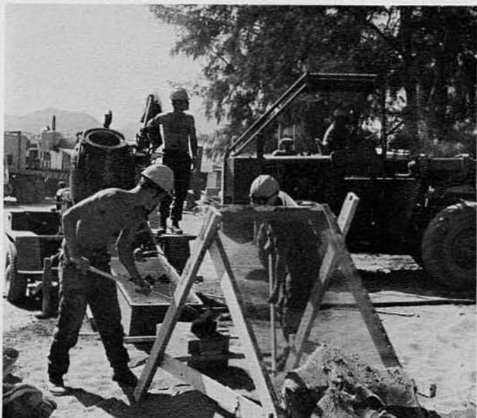
BU1 Viehmann, BUCN Langly and CECN Kirkman preparing to load the skip on the gunnite machine.
