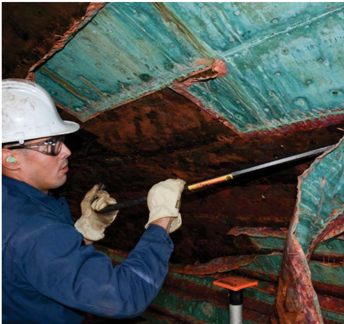
Seaman Jorge Ortiz, assigned to USS Constitution , pries a copper sheet away from the hull of Old Ironsides as a part of the restoration work being performed on the ship. Constitution is lined with 3,400 sheets of copper that are replaced every 15-20 years. U.S. Navy photo
